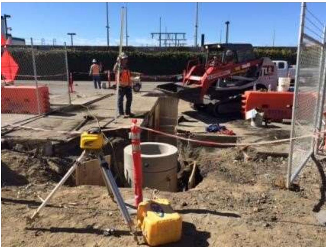
Figure 2: APEC conducting water and sewer line tie-in work on 23 rd Street, July 21, 2016.
