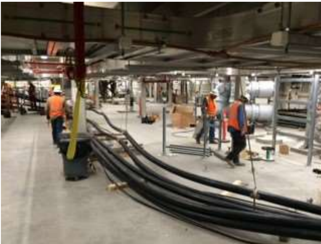
Figure 4: CCE installing infrastructure and electrical work in GIS building in the Potrero Switchyard, July 18, 2016.
