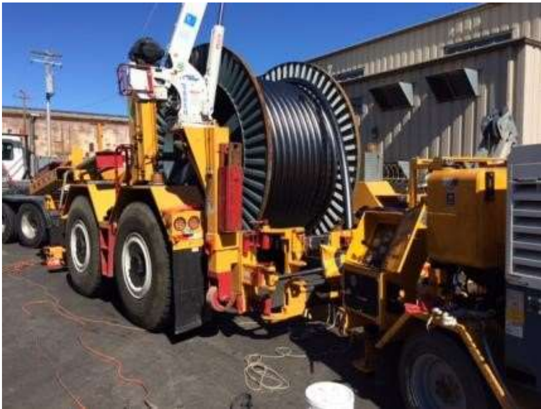
Figure 3: Sumitomo and NRE pulling cable at Duct Bank South on 23 rd Street, July 21, 2016.
