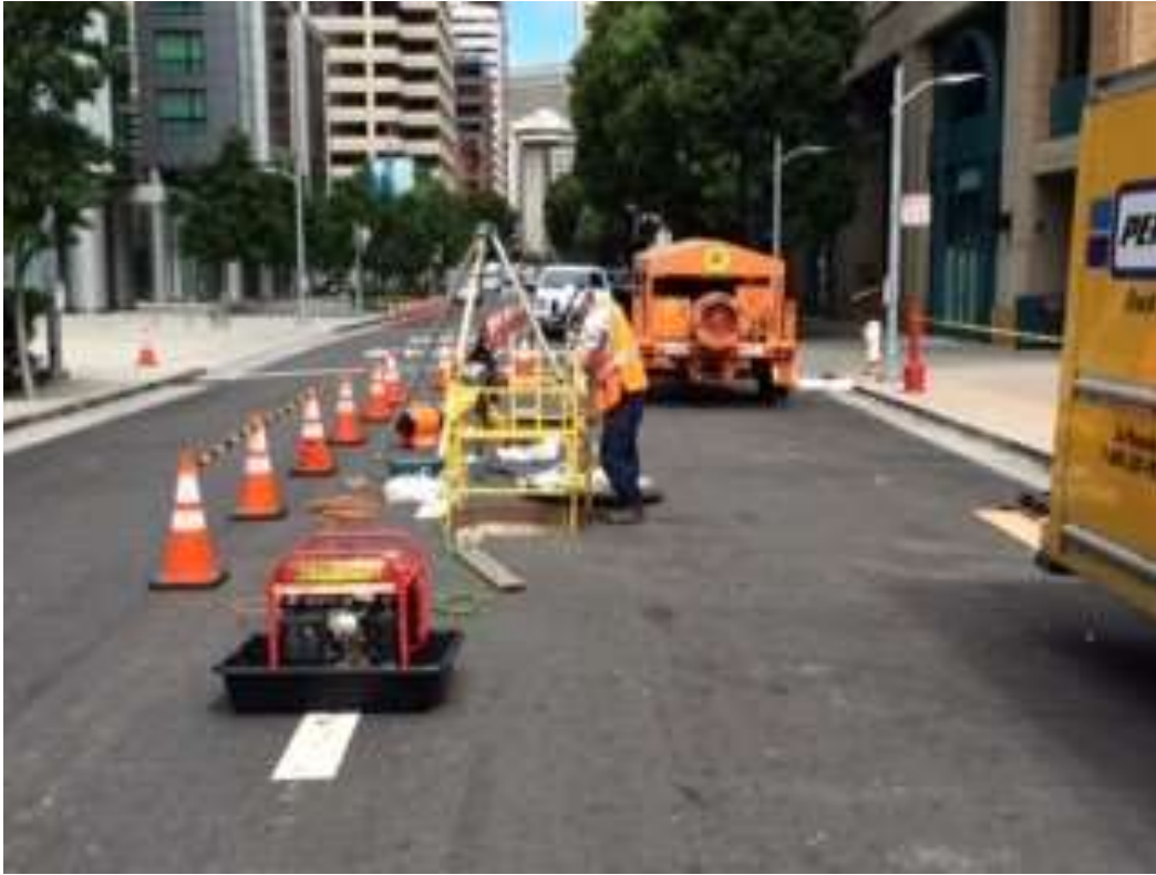
Figure 1: Sumitomo and NRE conducting racking inside the vault on Spear Street, July 18, 2016.
