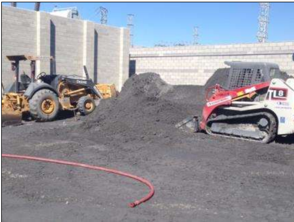
Figure 2 - APEC backfilled and compacted around GIS building at the Potrero Switchyard, September 27, 2016. Photo courtesy of PG&E.
