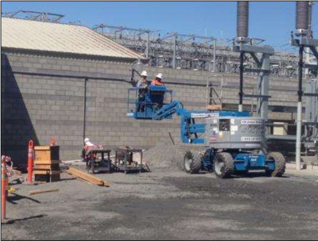
Figure 1 - CCE installing lights on perimeter wall at Potrero Switchyard, September 27, 2016. Photo courtesy of PG&E.
