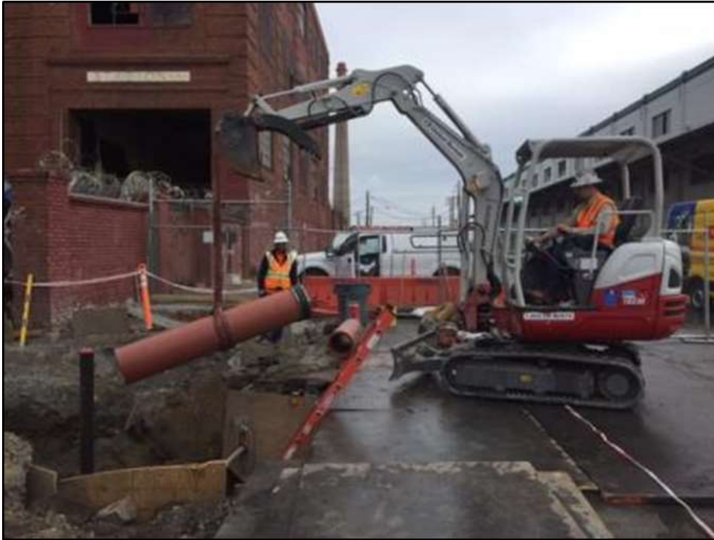
Figure 1 – APEC installing sewer pipe in southeast corner at Potrero Switchyard, October 3, 2016. Photo courtesy of PG&E.
