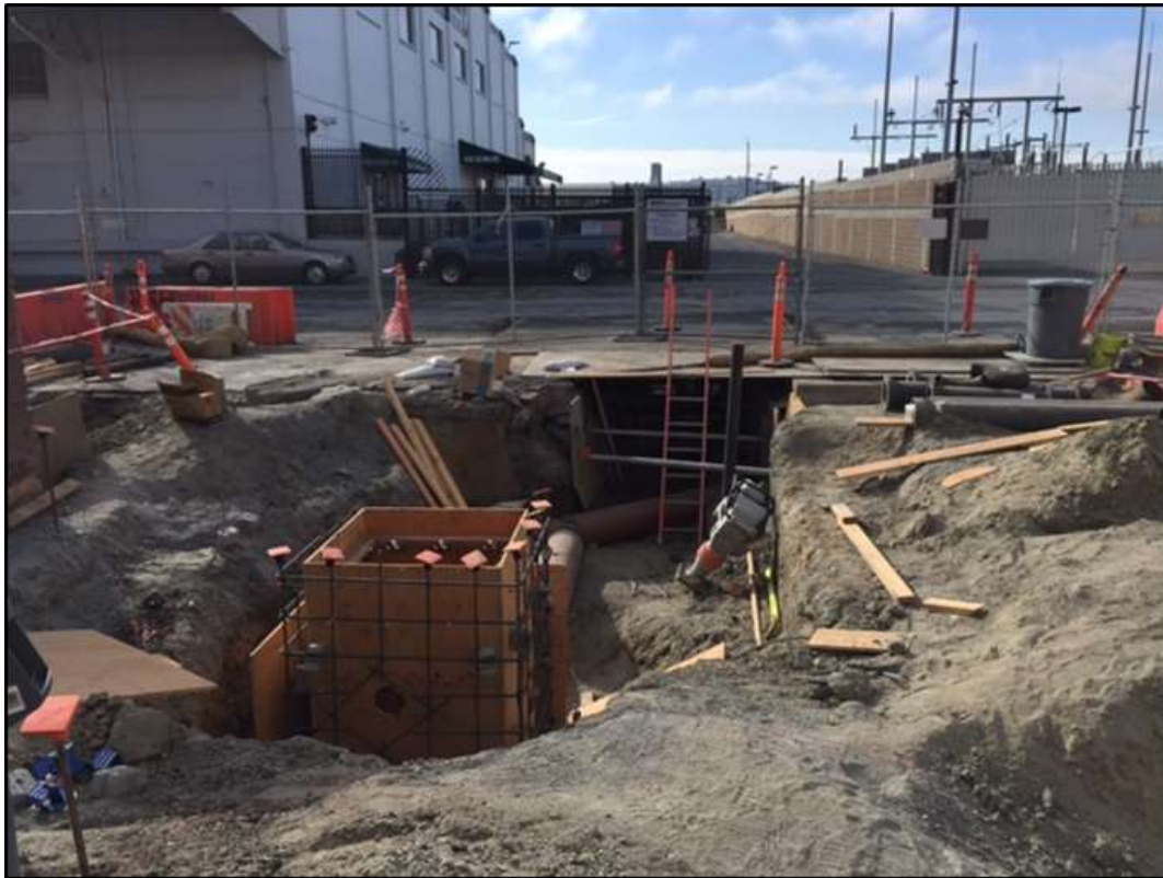
Figure 3 - APEC installing rebar and wood forms for sewer tie-in in southeast corner at the Potrero Switchyard, October 10, 2016. Photo courtesy of PG&E.
