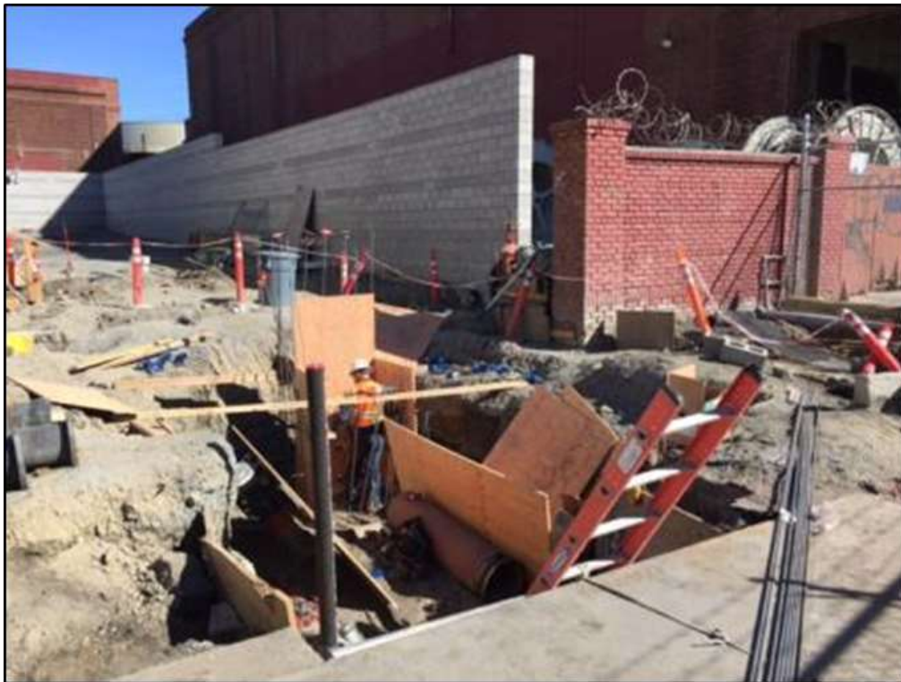
Figure 2 - APEC installing rebar and wood forms for sewer tie-in in southeast corner at the Potrero Switchyard, October 6, 2016. Photo courtesy of PG&E.
