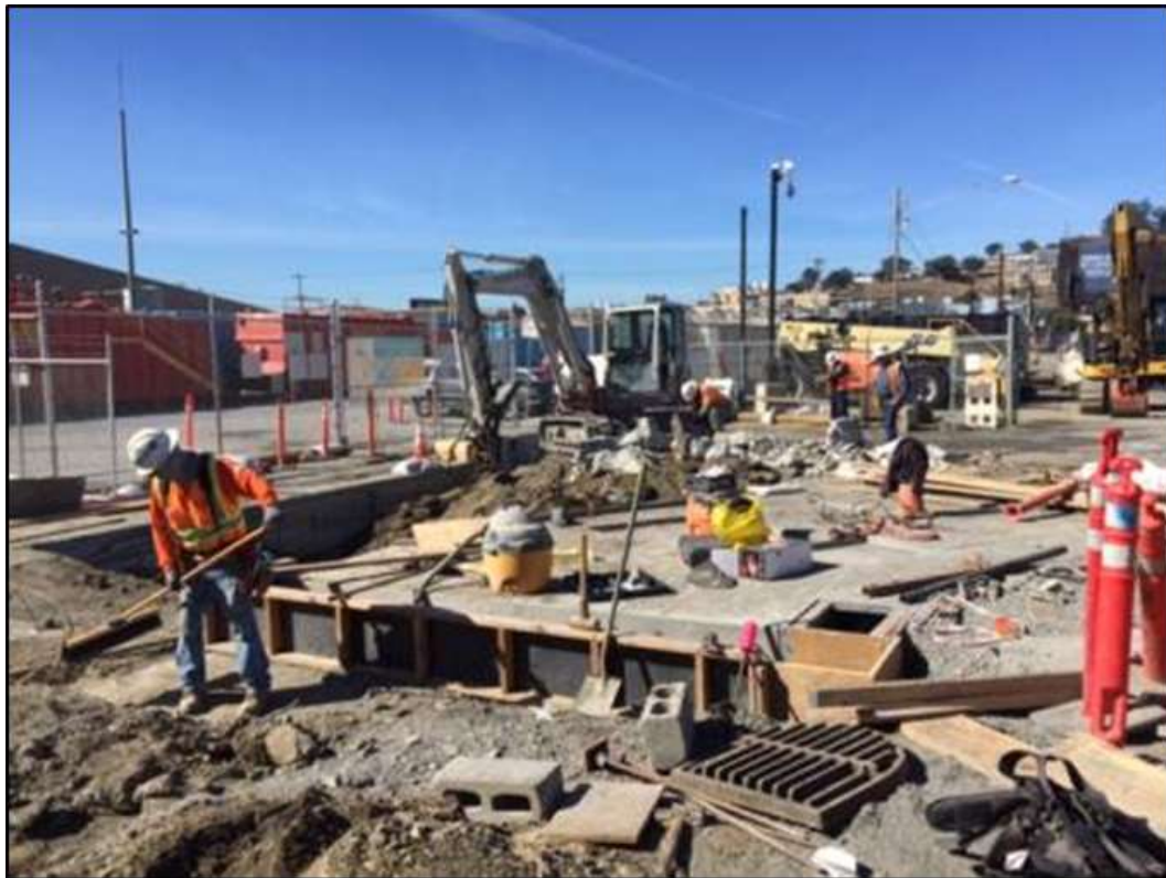
Figure 4 - APEC excavating for sewer tie-in in southwest corner at the Potrero Switchyard, October 6, 2016. Photo courtesy of PG&E.
