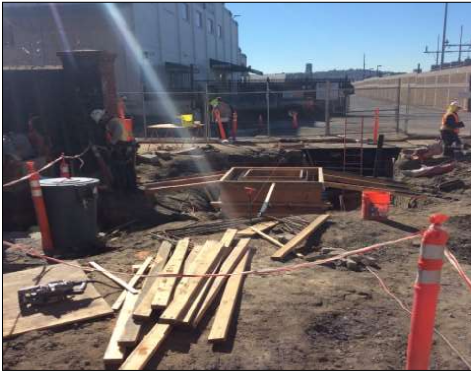
Figure 3 - APEC excavated and installed forms near the southeast corner of the GIS building for the water and sewer tie-in, October 20, 2016. Photo courtesy of PG&E.
