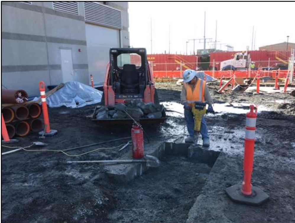
Figure 2 - APEC excavated west of the GIS building for surface drain installation at the Potrero Switchyard, October 17, 2016. Photo courtesy of PG&E.
