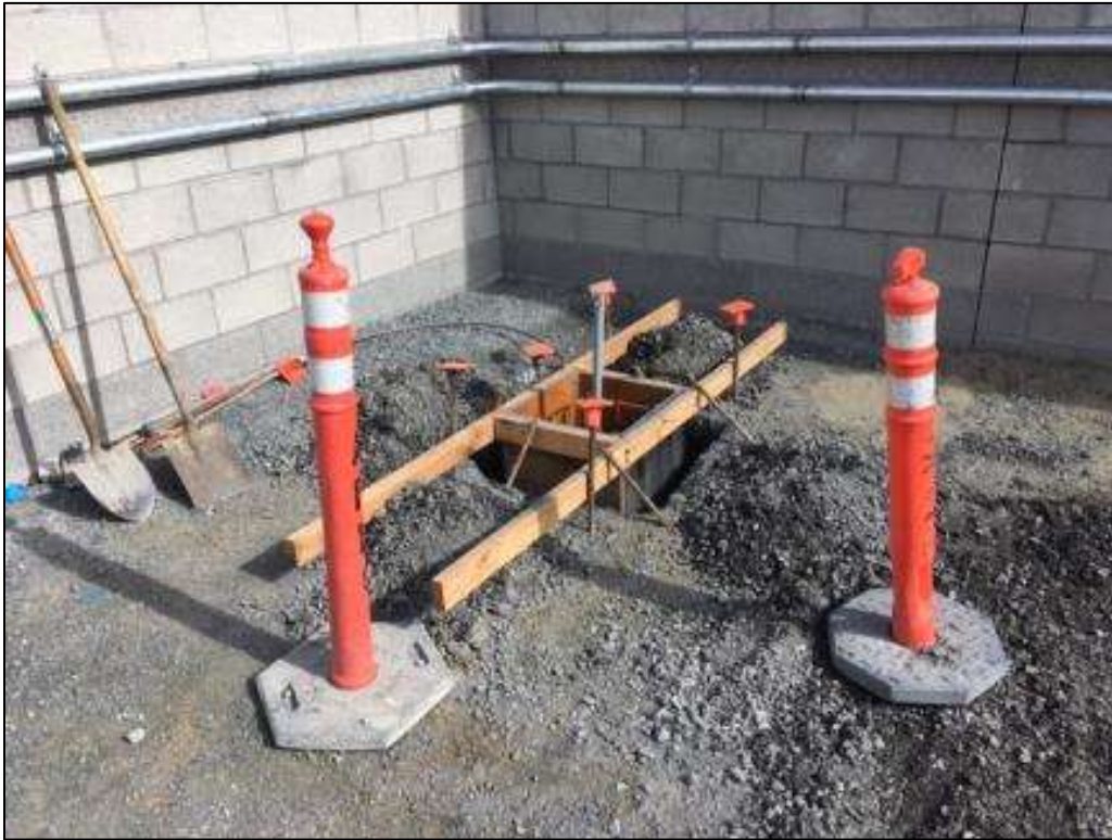
Figure 1 – CCE excavated, installed forms, and poured concrete for security beam tower foundations, November 7, 2016. Photo courtesy of PG&E.
