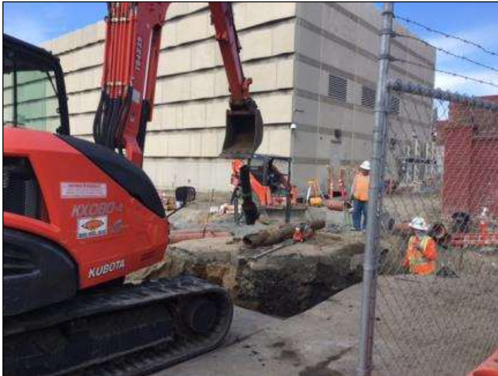
Figure 4 – APEC excavated and removed an abandoned pipe in the southeast corner of the yard for the water and sewer tie-in, November 10, 2016. Photo courtesy of PG&E.
