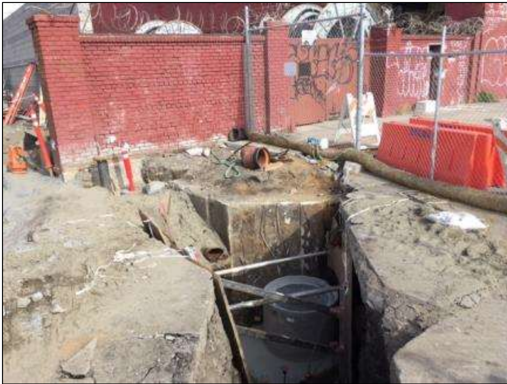
Figure 3 – APEC excavated and removed an abandoned pipe in the southeast corner of the yard relating to the water and sewer tie-in, November 7, 2016. Photo courtesy of PG&E.
