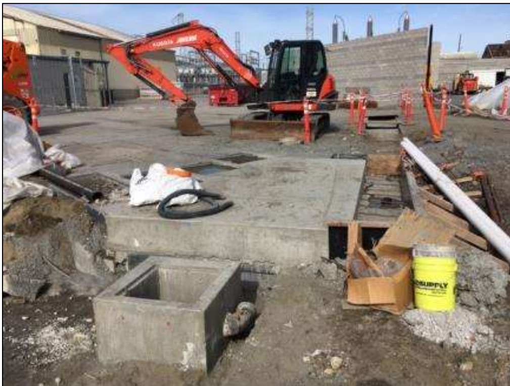
Figure 2 - APEC excavated near the southwest corner of the GIS building for the water and sewer tie-in, November 7, 2016. Photo courtesy of PG&E.
