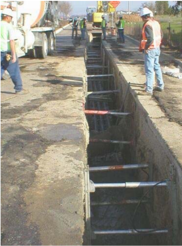
Trench in street. Conduit for individual transmission cables visible in center of photo.
