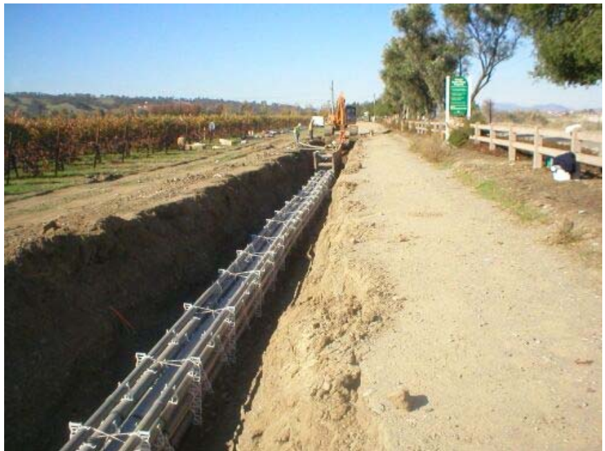
Double-circuit 230 kV underground cable conduit with spacers prior to pouring of concrete duct bank.
