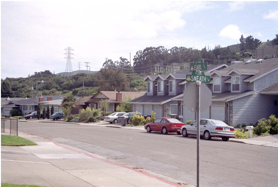
66. Sneath Substation and residences at Sneath Lane and Earl Avenue looking south
