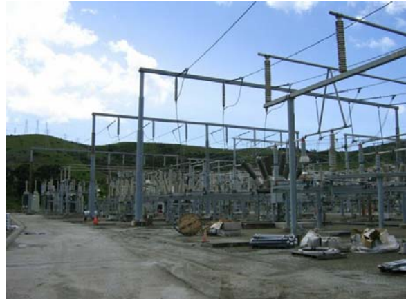
Figure 4-1. Martin Substation looking south (4-17-06)
