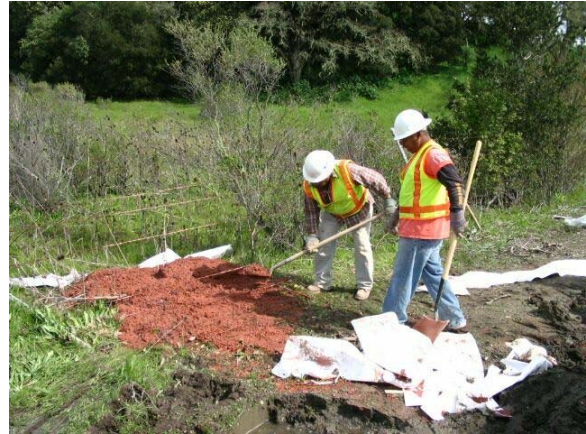
Figure 2-4. Crews cleaning up concrete spill (Segment 1, 3-16-05)
