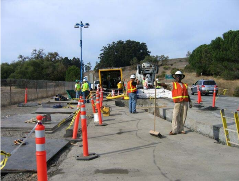
Figure 1 – Crews working at Manhole #1 stubouts and trench on south side, Segment 1, November 1, 2005
