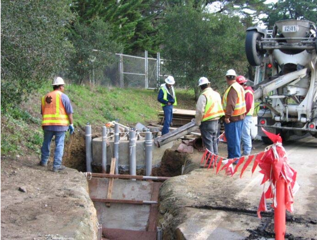
Figure 1 – Crews pouring cement slurry around the transition tower foundation on the north side of Crystal Springs Dam, Segment 1, January 10, 2006.
