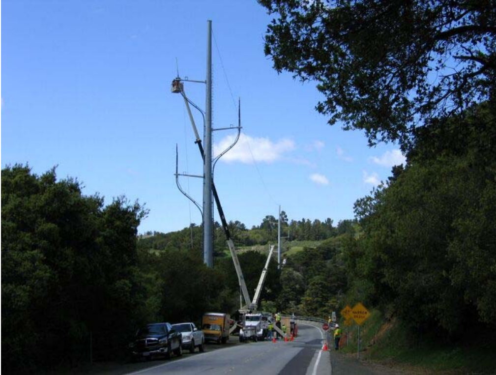
Figure 1 – Pot-head installation on tower at the south side of Crystal Springs Dam, Segment 1, April 17, 2006.
