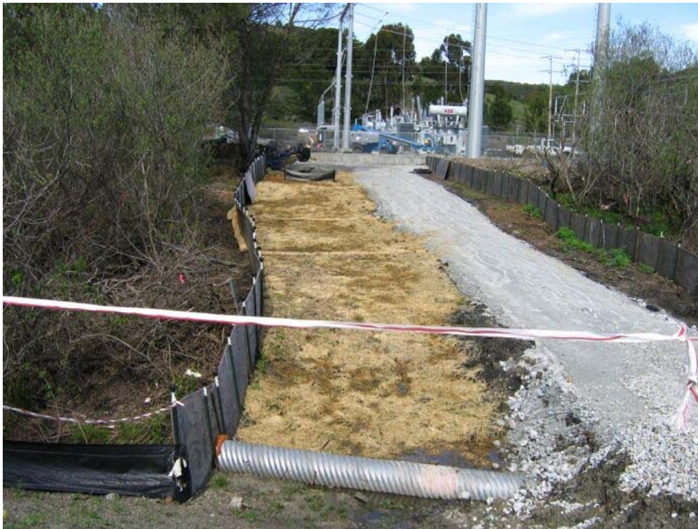
Figure 4 – New erosion controls on the right-of-way into the Jefferson Substation, April 13, 2006.
