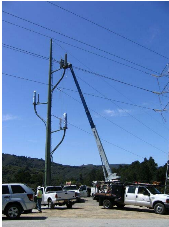
Figure 3 – Crews installing lightning arrestors and jumpers at Tower #70A, Segment 2 Overhead in the SFPUC Watershed, April 18, 2006.
