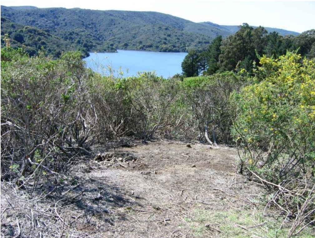
Figure 2 – Area where crews removed old Tower #75 concrete footings by hand, Segment 2 Overhead in the SFPUC watershed, April 13, 2006.
