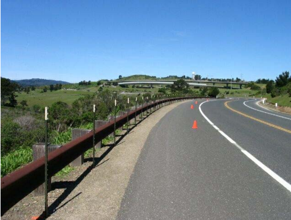
Figure 1 – Biological Exclusion Fence (green t-posts) being installed at Manhole #14 work area on west side of Cañada Road, Segment 1, March 25, 2005.
