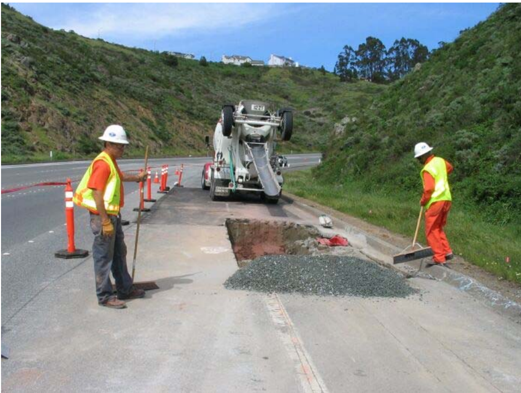
Figure 2 – Crews working at stub-out on West side of Manhole #67 on Guadalupe Canyon Parkway, Segment 5, March 25, 2005.
