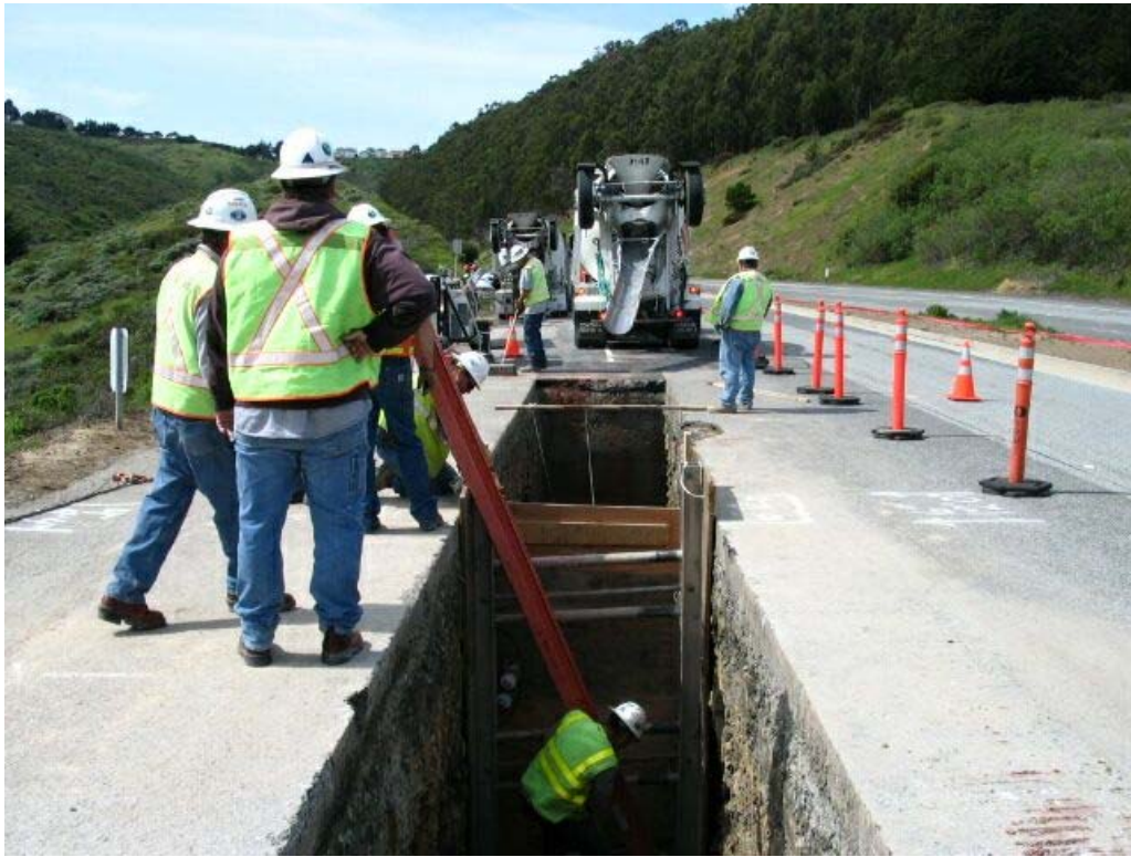
Figure 3 – Crews working at stub-out on east side of Manhole #69 on Guadalupe Canyon Parkway, Segment 5, March 25, 2005.
