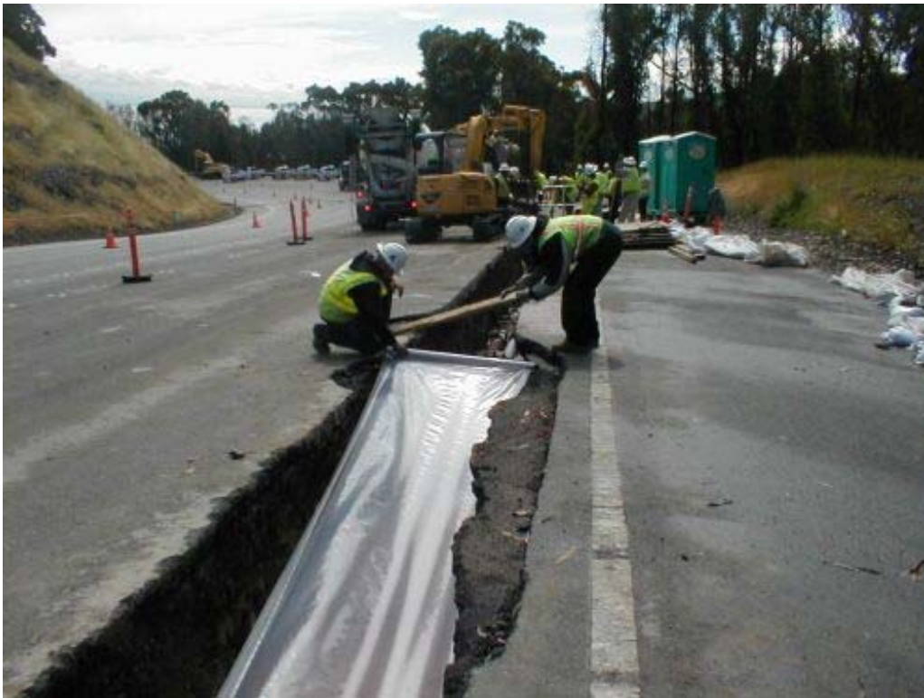
Figure 4 – Crews pouring cement slurry east of Manhole #72 on Guadalupe Canyon Parkway, Segment 5, April 28, 2005
