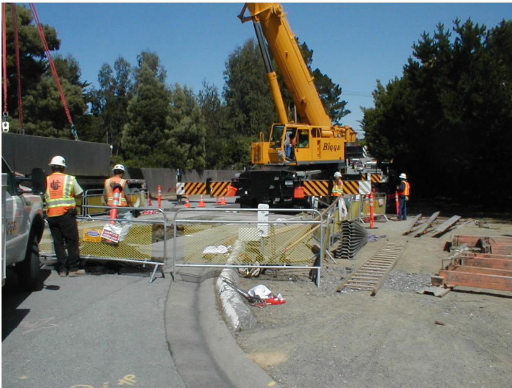
Figure 2 – Crews setting manhole vault at Manhole #33 on Skyline Boulevard, Segment 2 Underground, May 11, 2005
