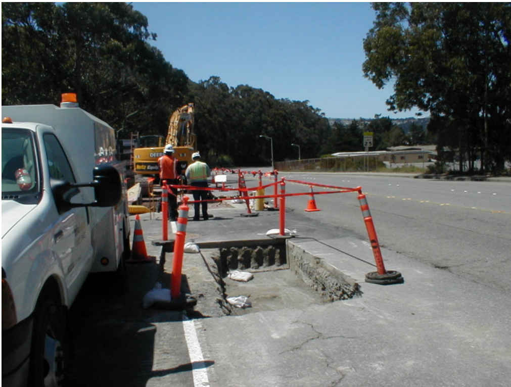
Figure 4 – Crews working on asphalt repairs at Manhole #66 on Guadalupe Canyon Parkway, Segment 5, May 10, 2005
