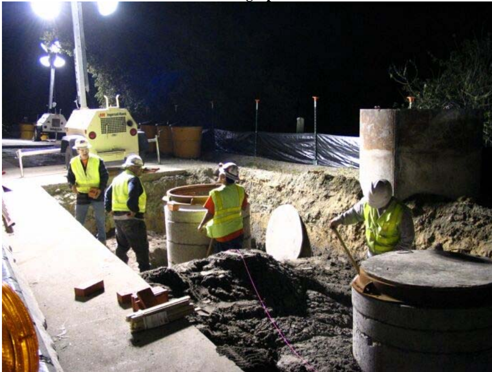
Figure 1 – Crews setting manhole rings at Manhole #21 in the Caltrans right-of-way on Skyline Boulevard, Segment 1, May 11, 2005
