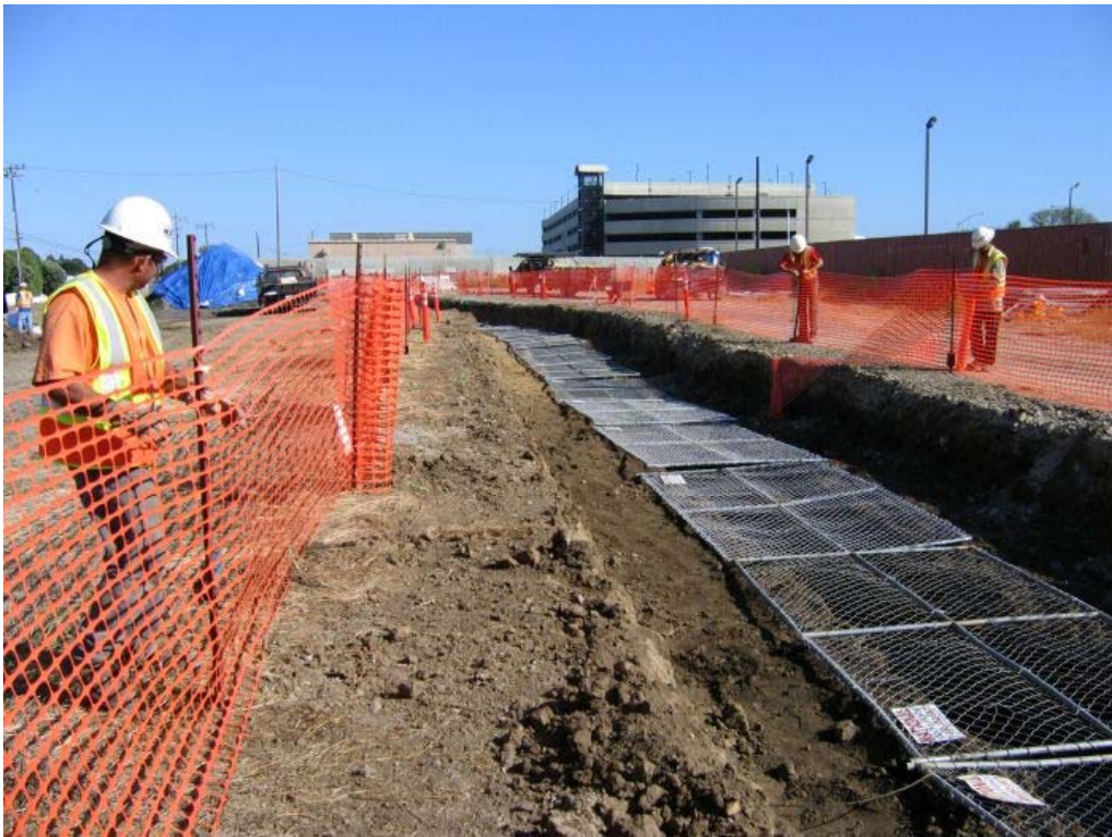
Figure 3 – Crews securing trenching area north of Manhole #48 in the BART right-of-way, Segment 4, June 1, 2005
