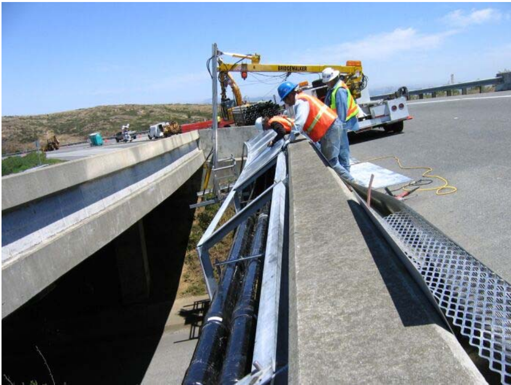
Figure 5 – Crew conducting bridge attachment on the top of San Bruno Mountain on Guadalupe Canyon Parkway, Segment 5, July 14, 2005.
