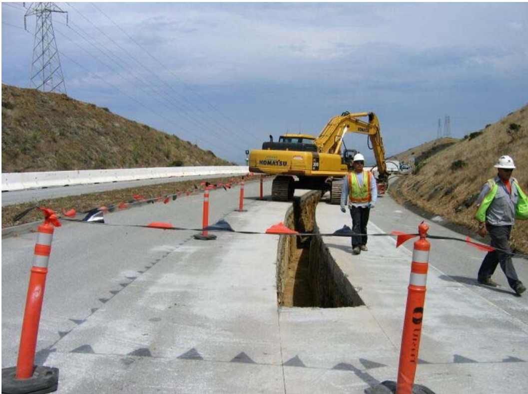
Figure 5 – Crews began trenching operations on the east side of San Bruno Mountain on Guadalupe Canyon Parkway, Segment 5, July 20, 2005.
