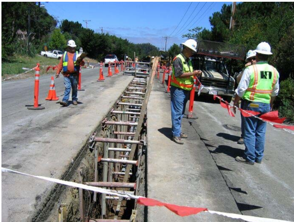
Figure 2 – Crews installing conduit on Skyline Boulevard south of Manhole #34, Segment 2 Underground, July 21, 2005
