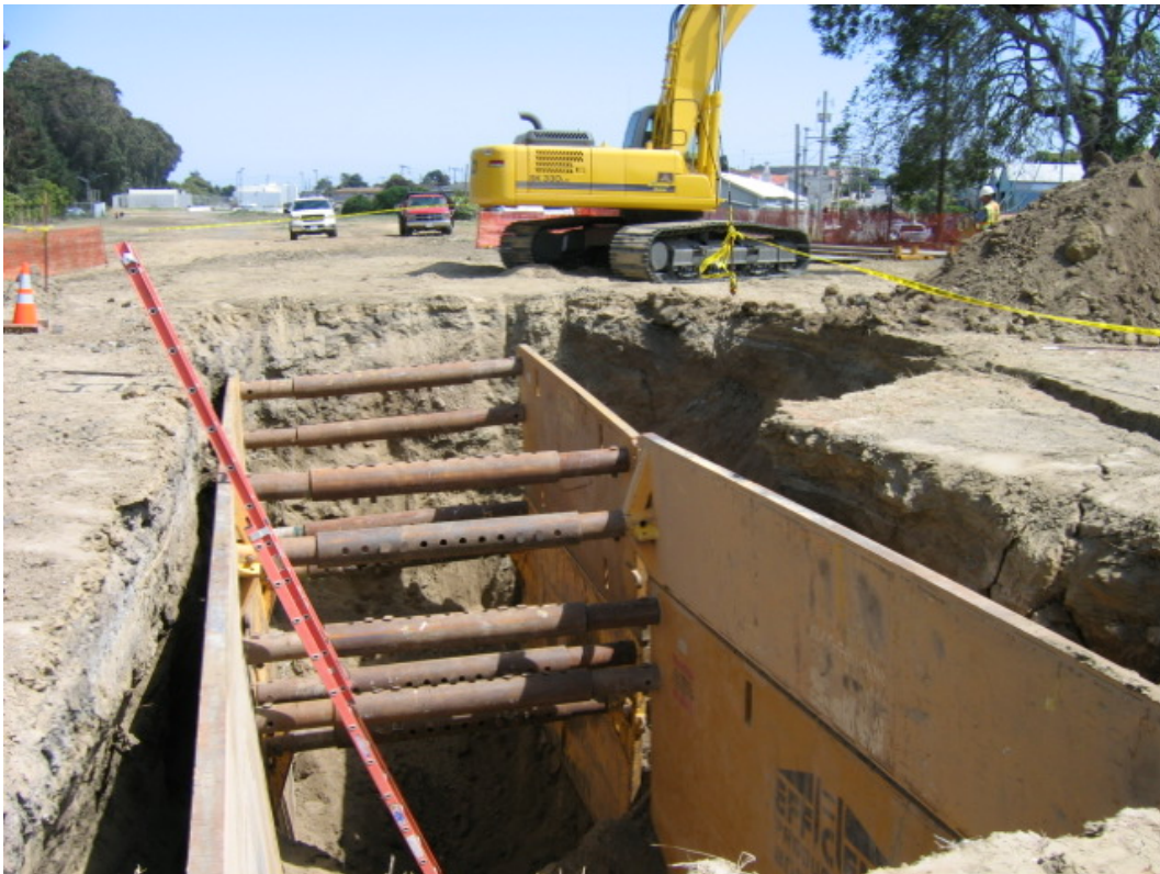
Figure 4 – Crews working at the entry bore pit on the south side of 12-Mile Creek, Segment 4, July 20, 2005
