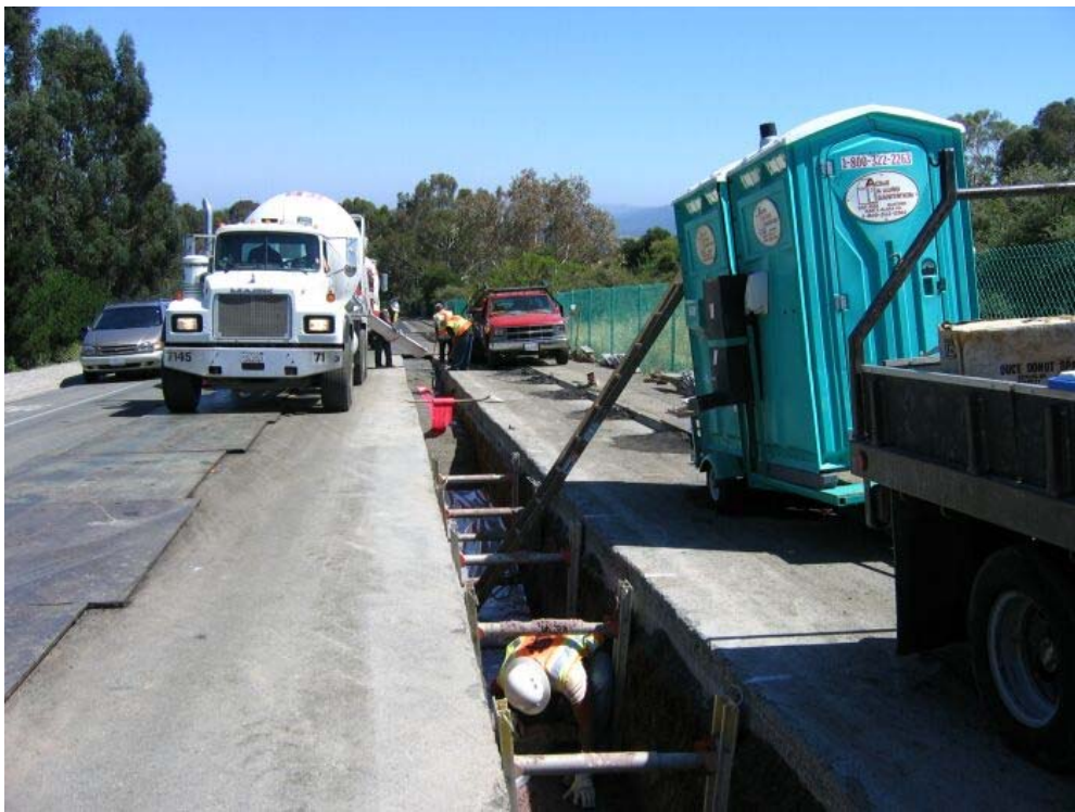
Figure 2 – Crews pouring cement slurry on Skyline Boulevard north of Manhole #28, Segment 2 Underground, July 28, 2005
