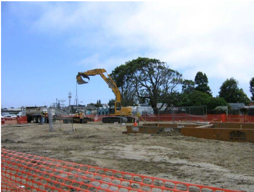
Figure 4 – Crews working at the entry bore pit on the south side of 12-Mile Creek, Segment 4, July 28, 2005
