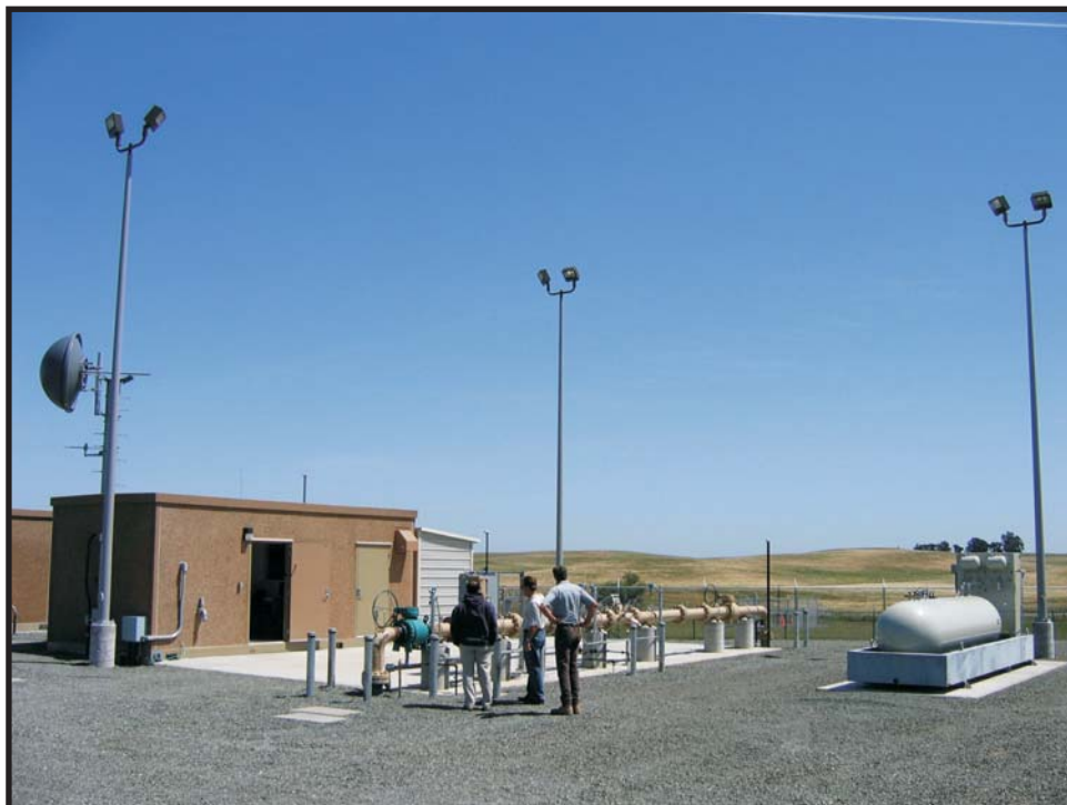
Metering Station constructed under the original Kirby Hills Natural Gas Storage Facility Project, April 26, 2007
