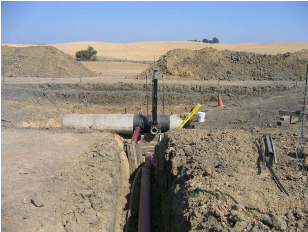
Figure 6 – PG&E ready to do hot-tap of their existing 32-inch pipeline just outside the Metering Station, September 28, 2006.
