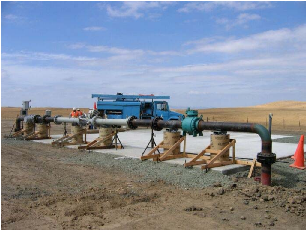
Figure 6 – PG&E working on pouring cement pipe supports at the Metering Station, October 3, 2006.
