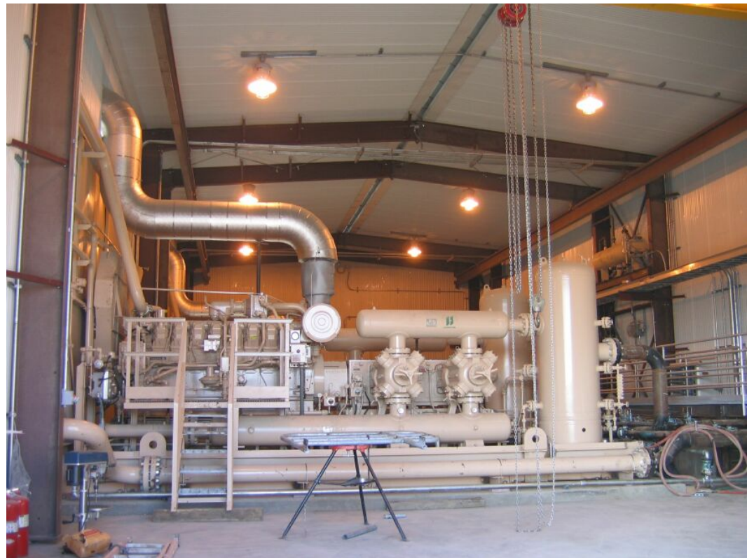
Figure 4-5. Inside the Compressor Building, 1-23-07
