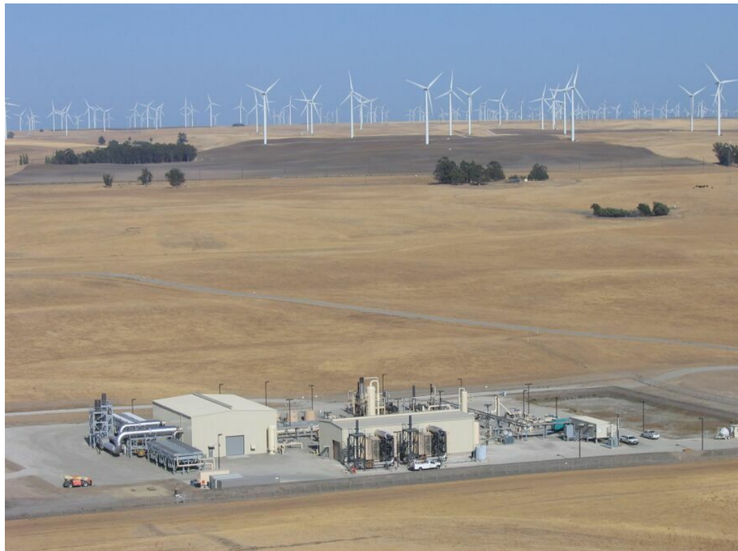
Figure 5-14. Completed Compressor Station for Phase II, 8-20-09
