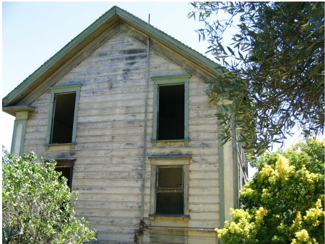
Figure 3-6. Abandoned House Used by Nesting and Roosting Birds, 6-22-06
