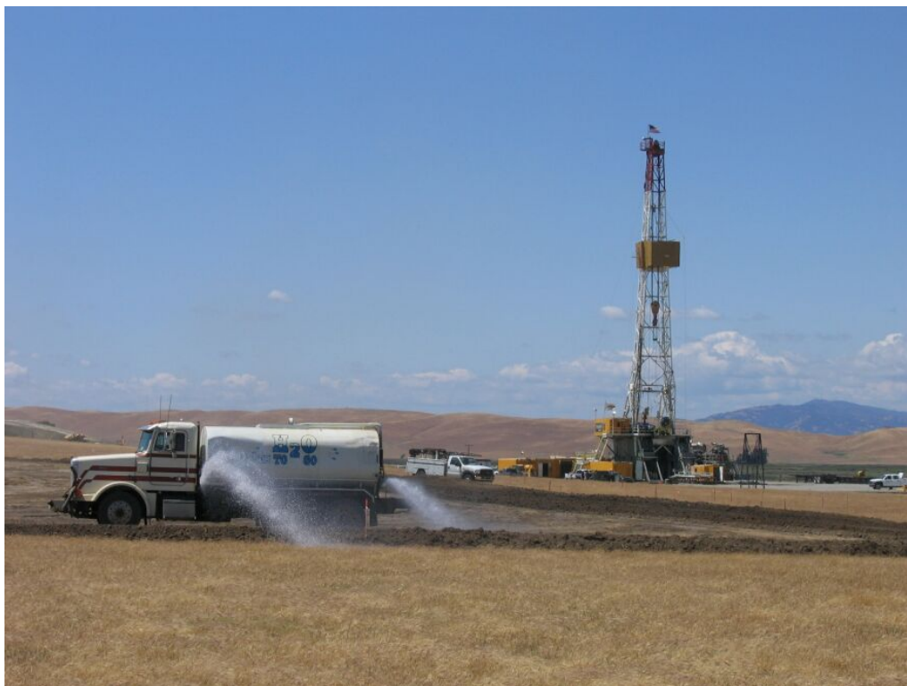
Figure 2 – Crews watering WS-21 pad. Drill rig at WS-22 in the background, May 29, 2008.
