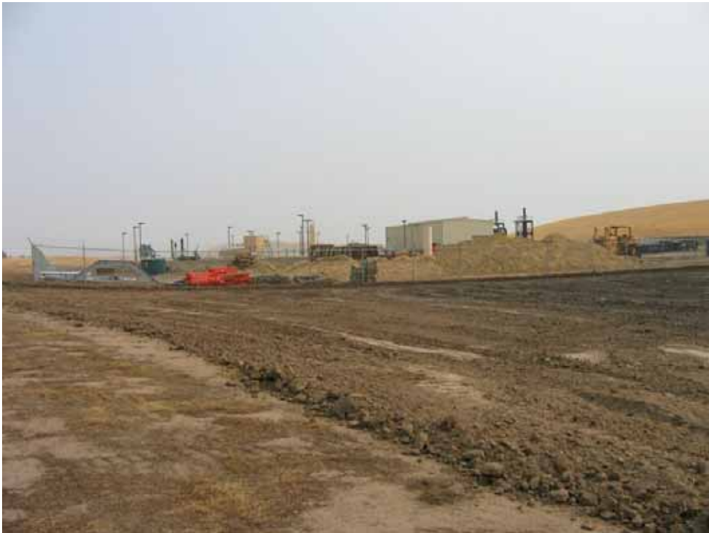
Figure 2 – Staging area/work area on the north side of the Compressor Station, July 10, 2008.
