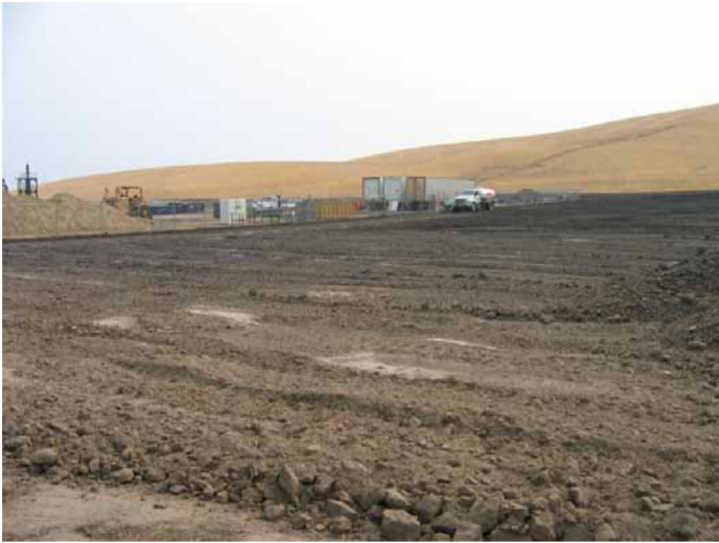
Figure 3 – Staging area/work area on the north side of the Compressor Station, July 10, 2008.
