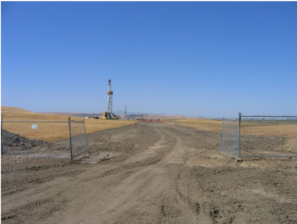
Figure 3 – Pipeline right-of-way trench backfilled from the Compressor Station to WS-21 well pad, August 28, 2008.
