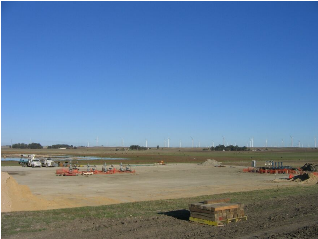
Figure 2 – Well-head piping at well site 22 (WS-22), November 21, 2008.
