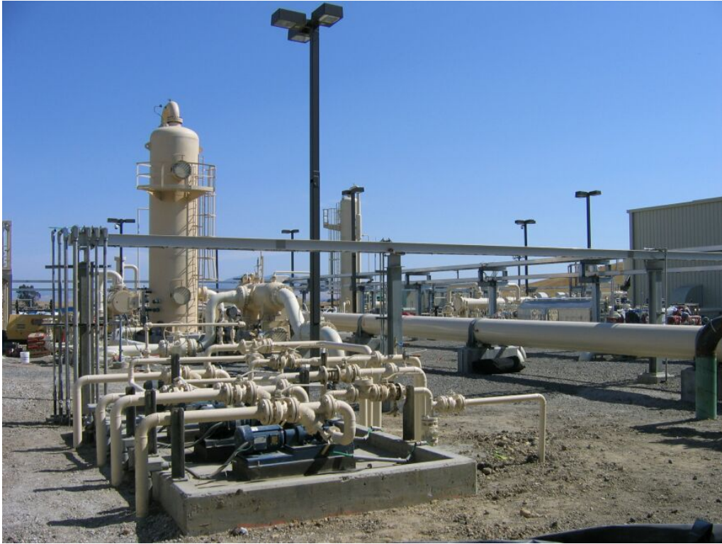
Figure 1 – Compressor Station piping, May 28, 2009
