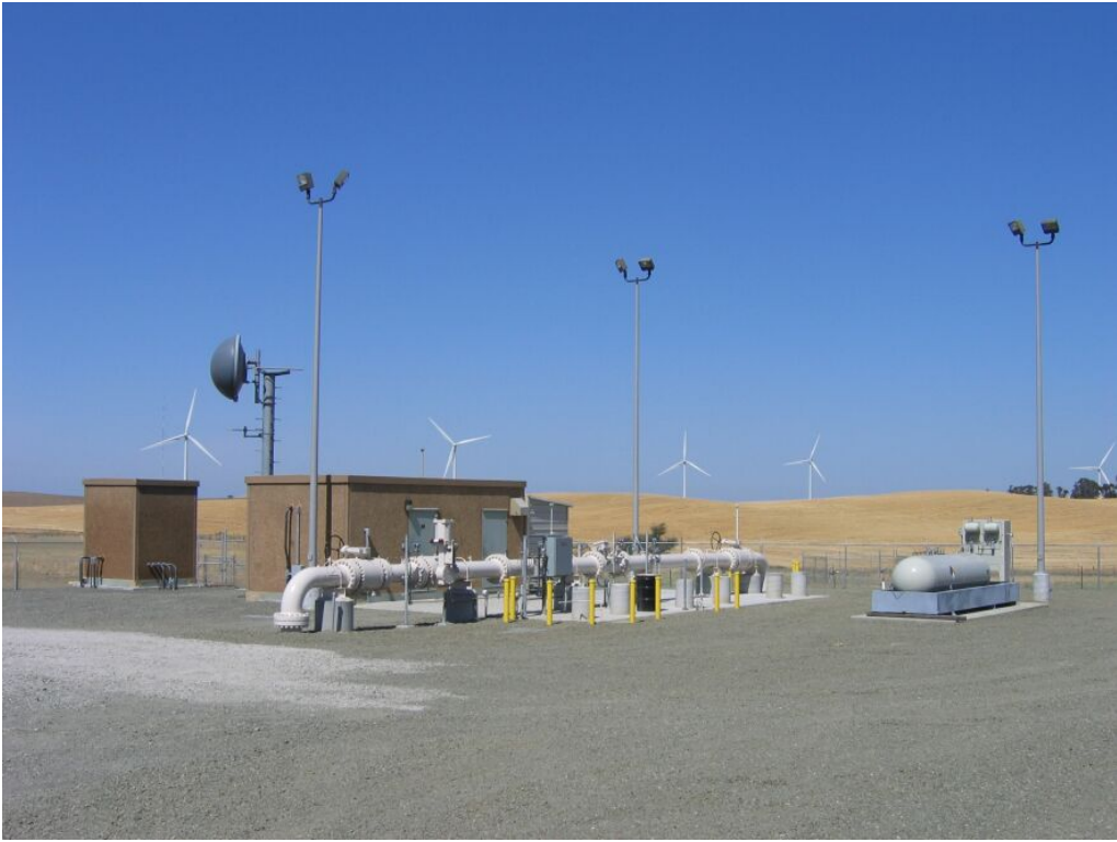
Figure 5 – Metering Station work complete, July 9, 2009
