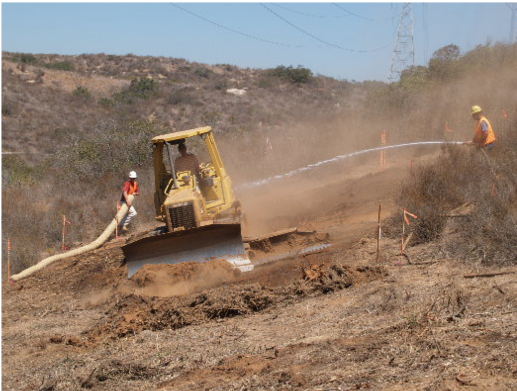
Figure 4 – Grading work started at Site 321 above Steele Canyon High School. The Essex EI worked with the water truck operator to improve dust control.
