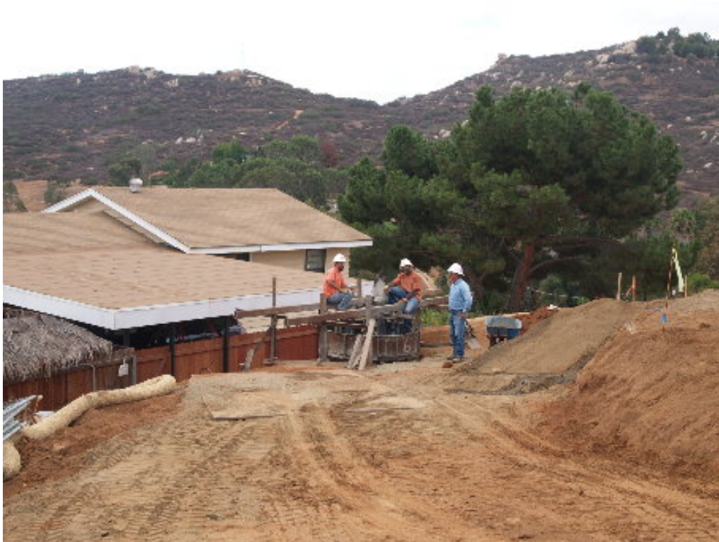
Figure 1 – The PAR crew at Tower Site 1270 started the concrete pour adjacent to the carport.
