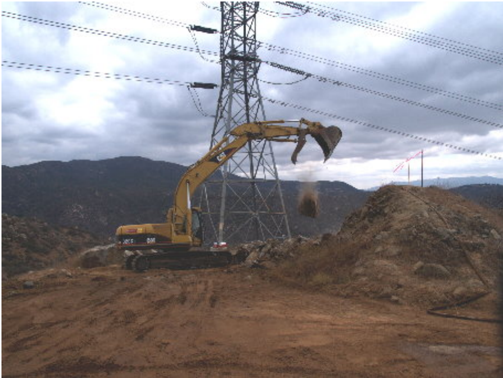
Figure 5 – The excavator operator at Tower Site 611 moved rock from the pad and loaded it in trucks for removal.
