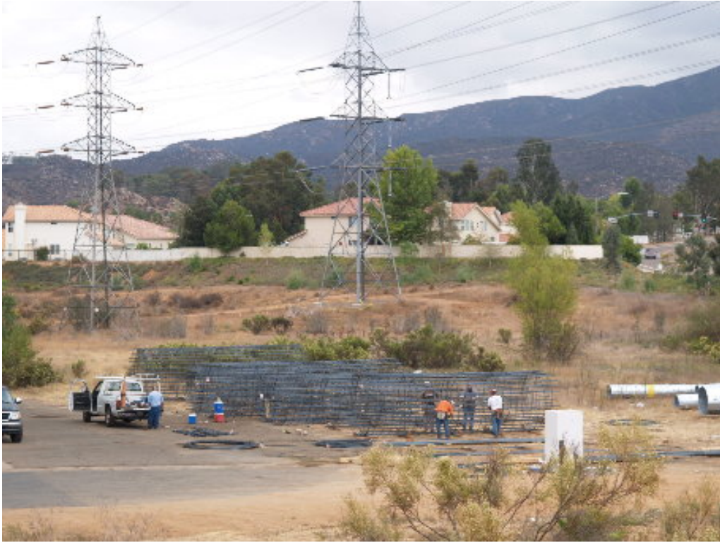
Figure 3 – Ironworkers built cages at the staging area adjacent to the special-needs school. The cages will be placed in the completed bore holes.
