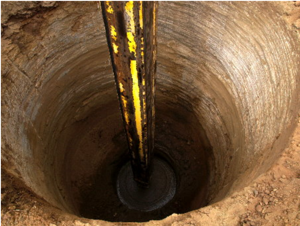
Figure 4 – The boring crew at Tower 990 encountered dense rock and drilling proceeded slowly. Water is used to keep the drill head cool during boring.
