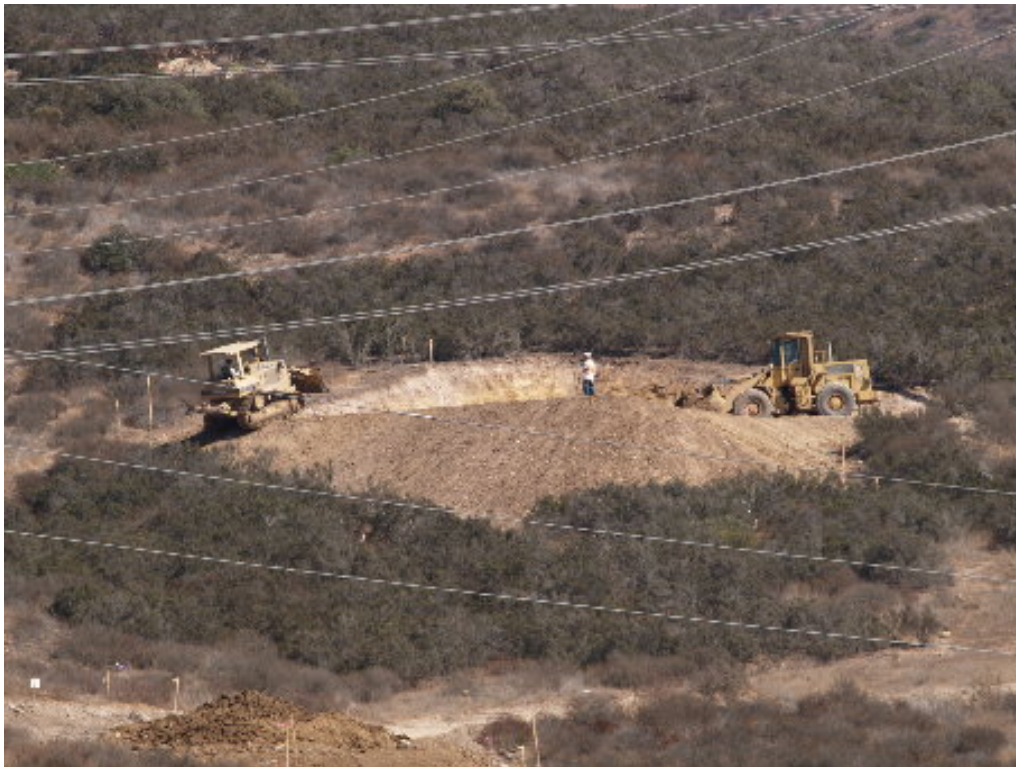
Figure 2 – The grading crew worked to finish the pad at Tower Site 10. The spoil pile below is material imported to build up Tower Site 5/7.
