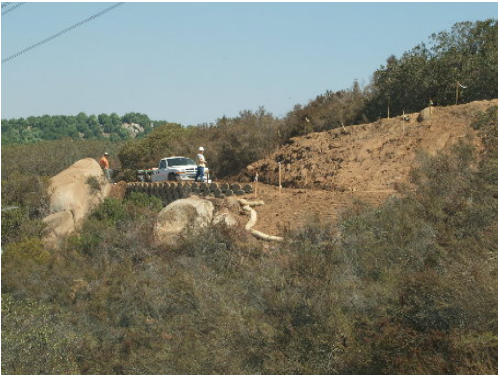
Figure 6 – The crew at Tower Site 932 completed the retaining wall and installation of the erosion control devices.
