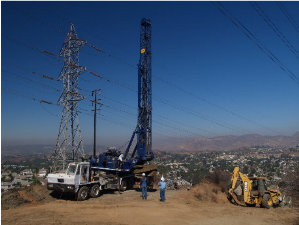
Figure 3 – The drilling crew moved back from Tower Site 925A to 925 to remove a bad batch of concrete from the hole.
