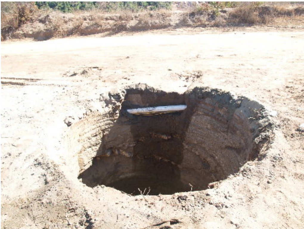
Figure 4 – A foreign utility was encountered during the drilling at Tower Site 925A. The water is from cooling the drill head and not from the PVC pipe.
