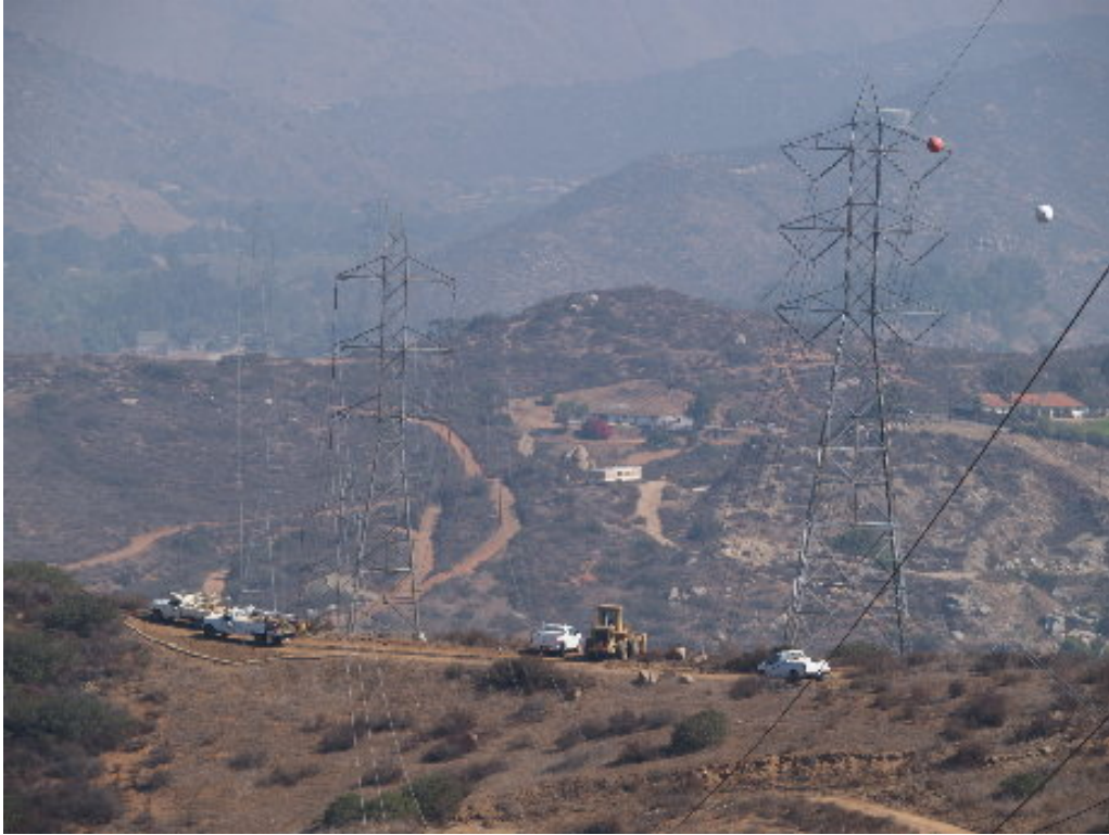
Figure 1 – The grading crew finished Tower Site 232 and moved down the hill to start Tower Site 242.
