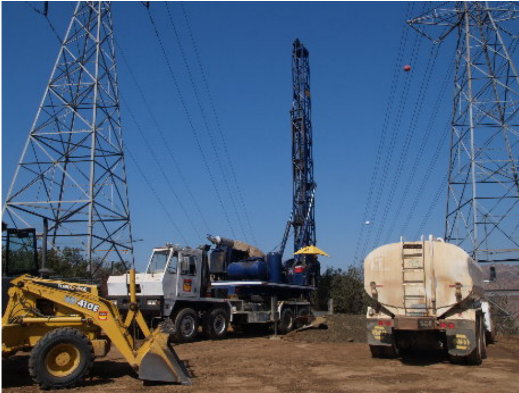
Figure 5 – The second drilling crew worked near houses at the tower site on Vista Rodeo.
