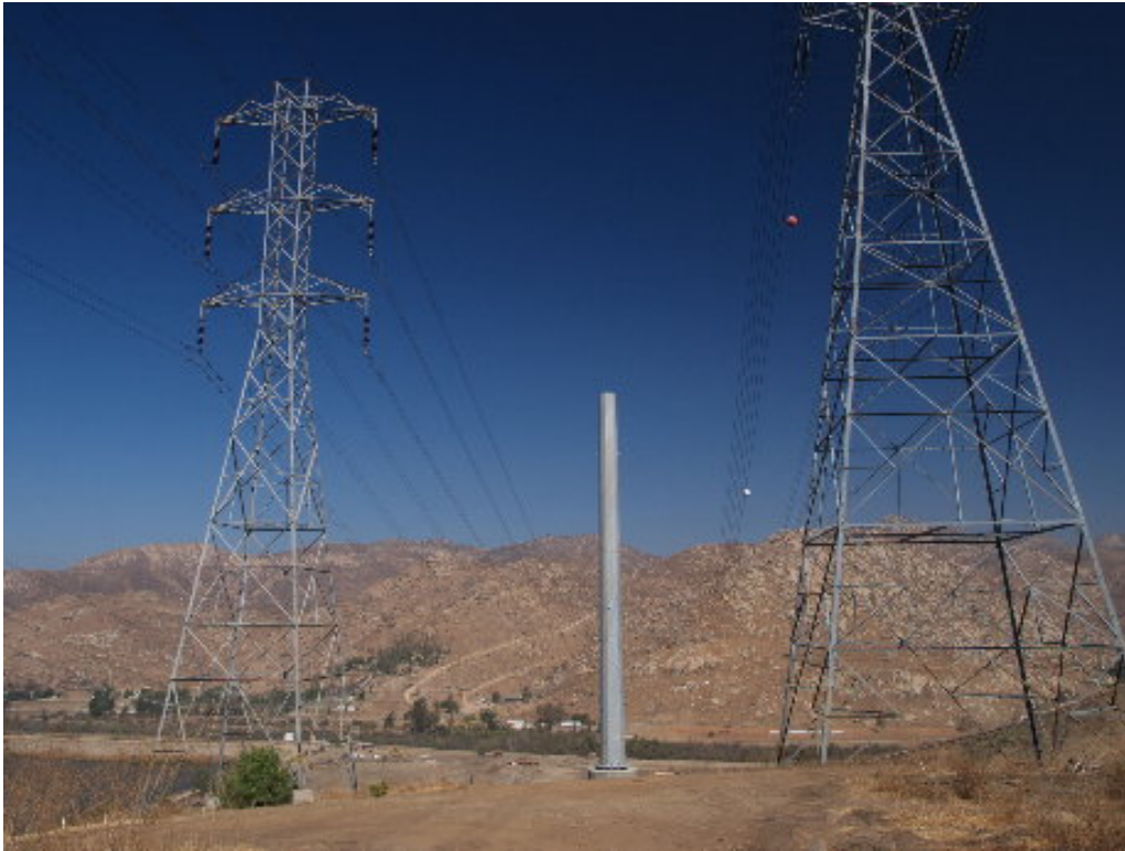
Figure 3 – The PAR crew erected the lower section of the pole at Tower Site 635.
