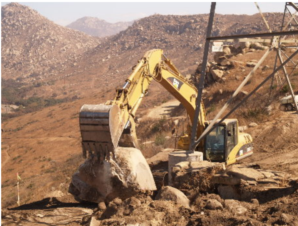
Figure 1 – The grading crew worked carefully to move large boulders at Tower Site 1180 without allowing spoils or rock to roll off the ridge line.
