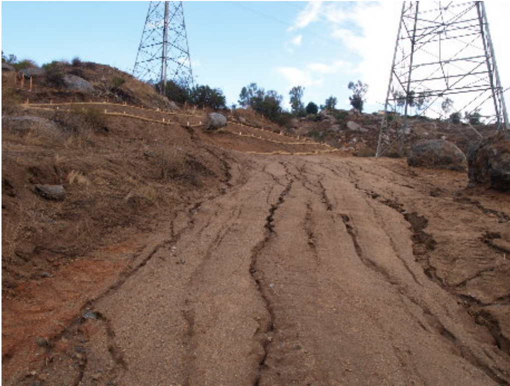
Figure 5 – The water bars at Tower Site 440 were completely washed away and sediment flowed onto the public right-of-way and into the storm drain.
