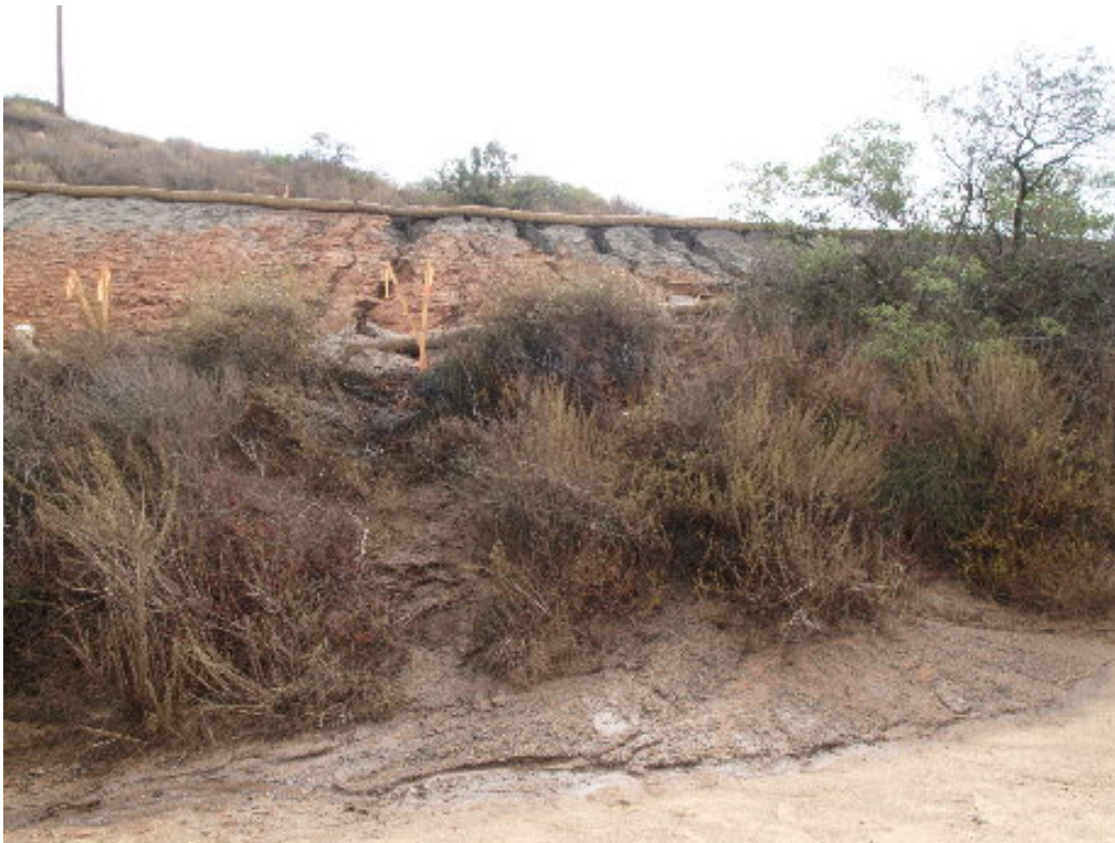
Figure 6 – The straw waddles at Tower Site 325 were undercut as run-off from the access road flowed over the crane pad and sediment flowed down through the vegetation.
