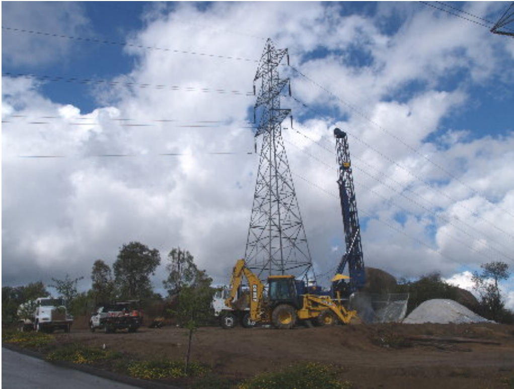
Figure 3 – The drilling crew continued on the foundation at Vista Rodeo during the subject week, stopping only briefly for heavy rainfall.
