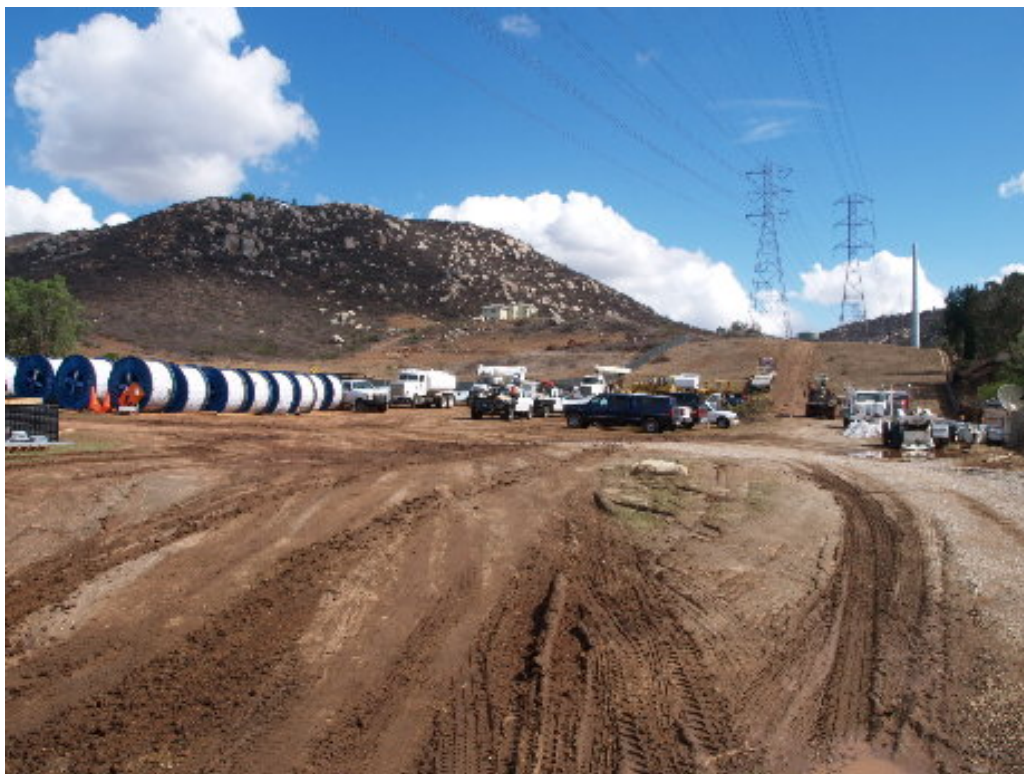
Figure 1 – The transmission line contractor worked at the Summit Road yard. Note the lower tower section erected on the upper right of the photograph.
