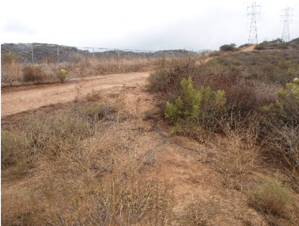
Figure 4 – Sediment flowed off the access road into the adjacent coastal sage scrub habitat. Water bars were excessively steep and lacked sediment traps.
