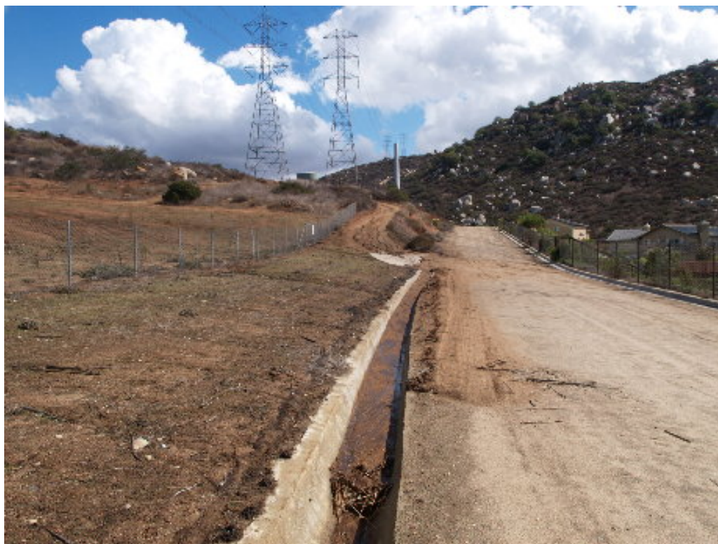
Figure 2 – Sediment from Tower Site 1310 flowed into an adjacent concrete V-ditch.
