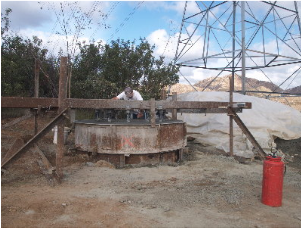
Figure 3 – The drilling crew finished the foundation at Vista Rodeo and a worker finished the foundation surface after the concrete pour.
