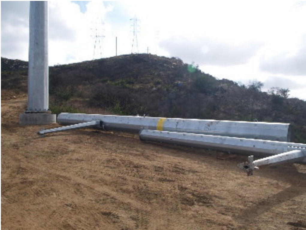
Figure 4 – The upper sections of the poles at Tower Site 925A are on-site for raising during the weekend outage covered in Variance Request #6.
