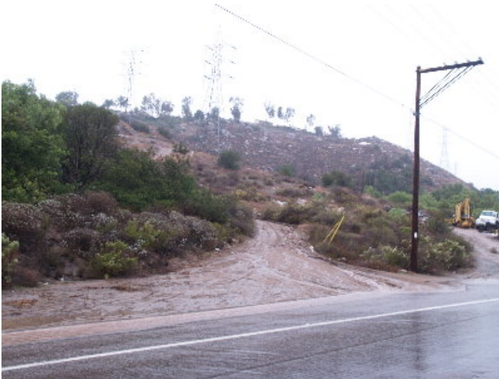
Figure 6 – The water bars at Tower Site 440 were completely washed away and sediment flowed onto the public right-of-way and into the storm drain.
