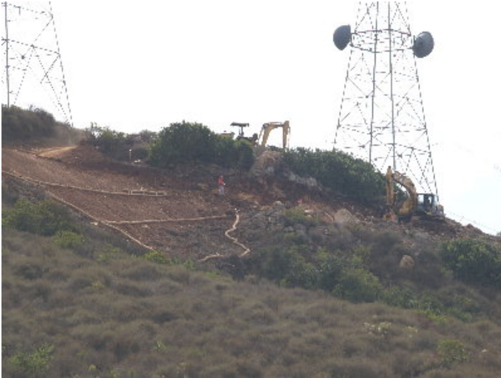
Figure 1 – The grading contractor returned to Tower Site 80 to remove spoils while the access roads were passable. The straw waddles were installed at too steep an angle.
