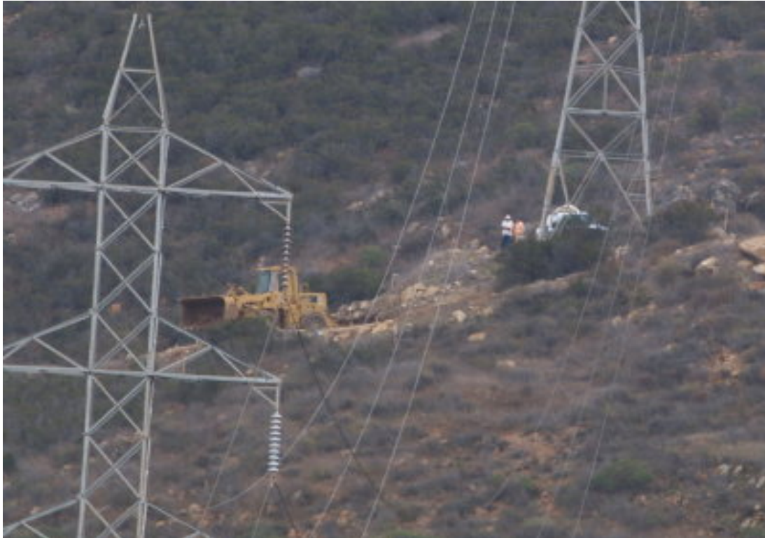
Figure 2 – A grading crew worked to repair storm damage and improve BMPs at Tower Site 151.
