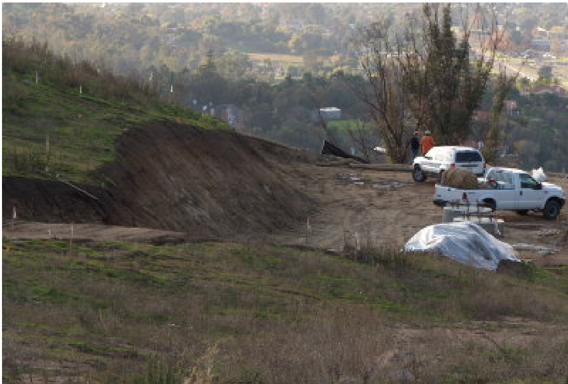
Figure 4 – The cut slope at Tower Site 797 is primarily bedrock and cannot be stabilized by matting.
