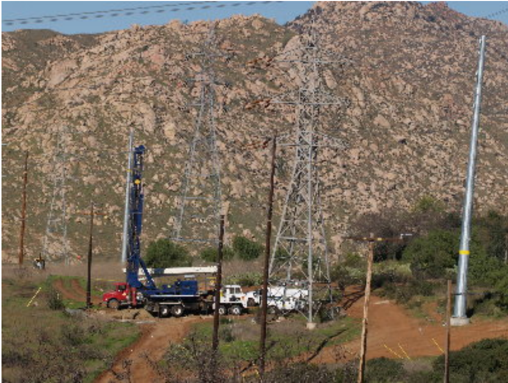
Figure 3 – A drill continued work above the Los Coches Substation at Tower Site 1140.
