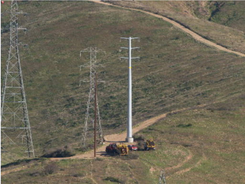
Figure 1 – Cable puller and reel truck set up north of Santee Lakes during stringing operation.
