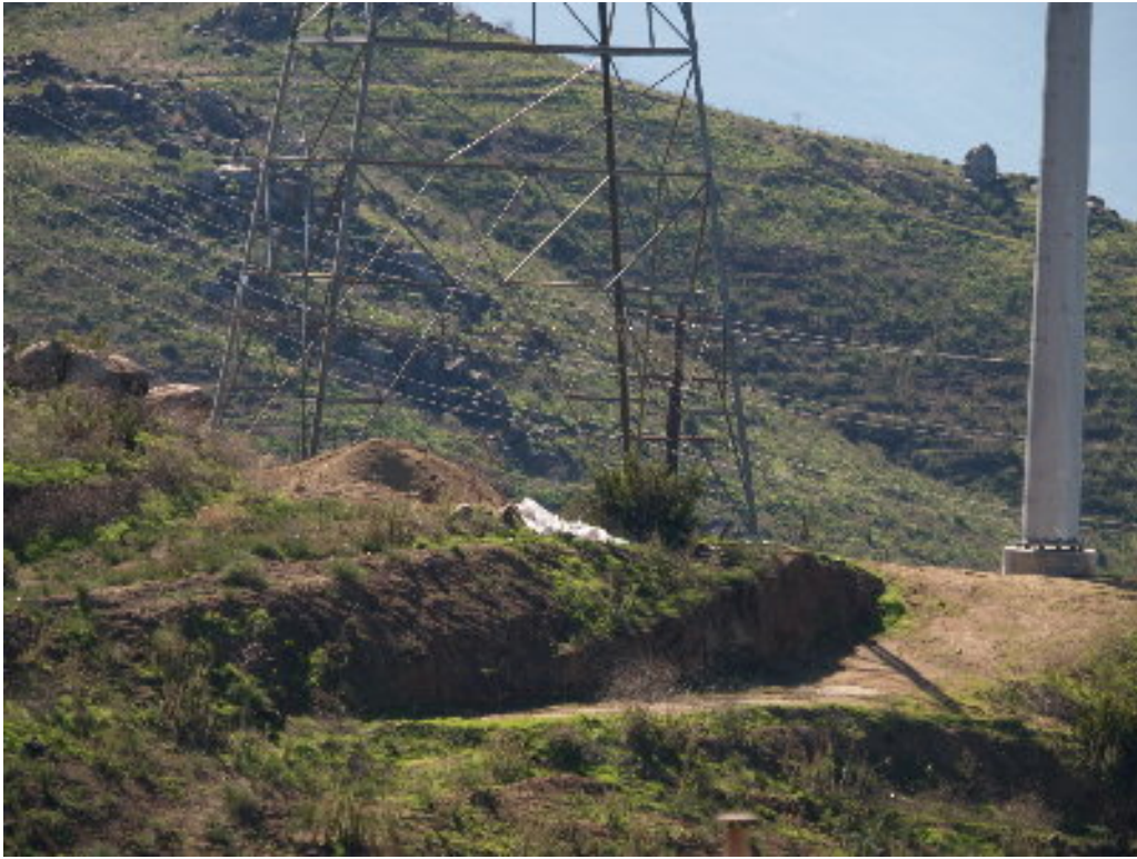
Figure 5 – The Union reseeding crew is waiting for other contractors to remove spoil piles and repair most of the pad locations before proceeding with permanent restoration.
