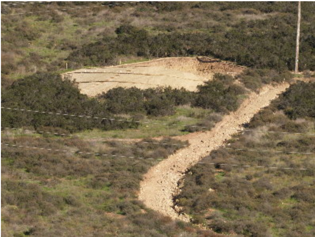
Figure 4 – The Union crew reseeded Tower Site 10 east of the Miguel Substation. Note the condition of the access road following the heavy rainfall.
