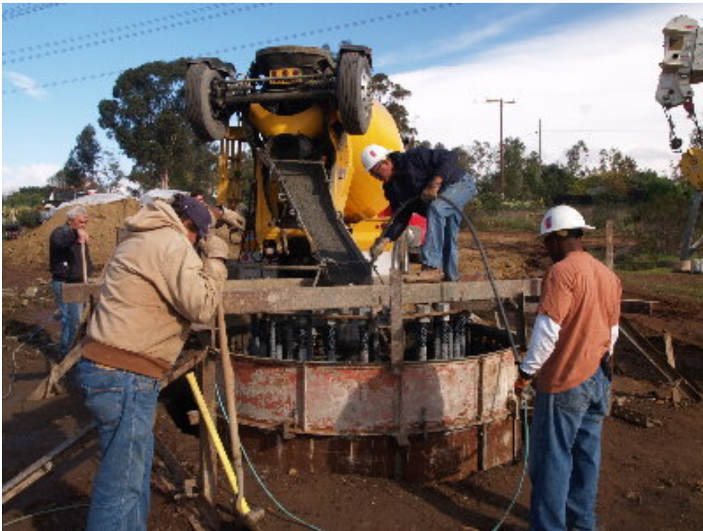
Figure 6 – The PAR crew worked to pour concrete in the foundation forms at Tower Site 1140.
