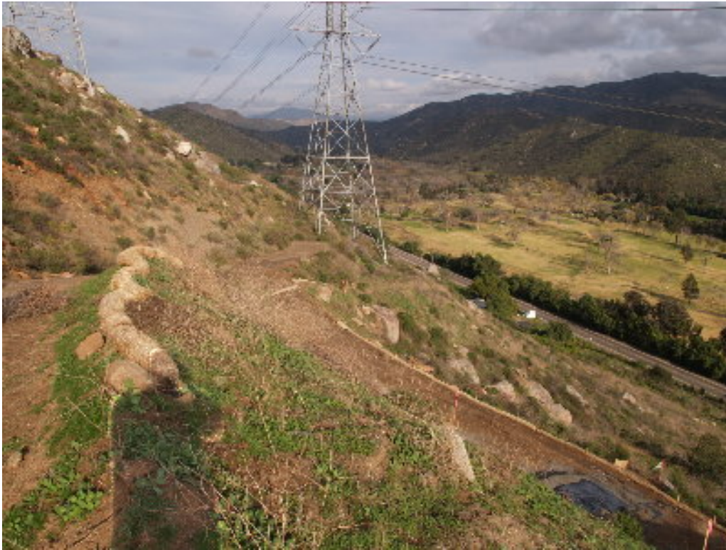
Figure 7 – Location of Tower Site 481 (excavation covered with black plastic on bottom right) relative to existing lattice towers. Note the steep side slope.
