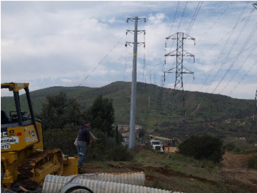
Figure 4 – The PAR stringing crew worked to anchor the guy wire from the steel pole to the bulldozer to prevent the pole from bending under the pull of the cable.
