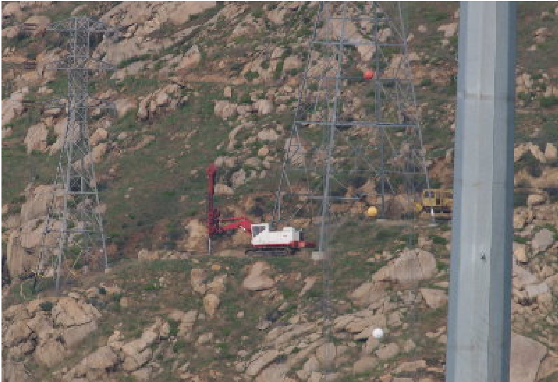
Figure 5 – The Low Drill moved to Tower Site 1160 and started drilling during the end of the previous week. Work continued on December 7.
