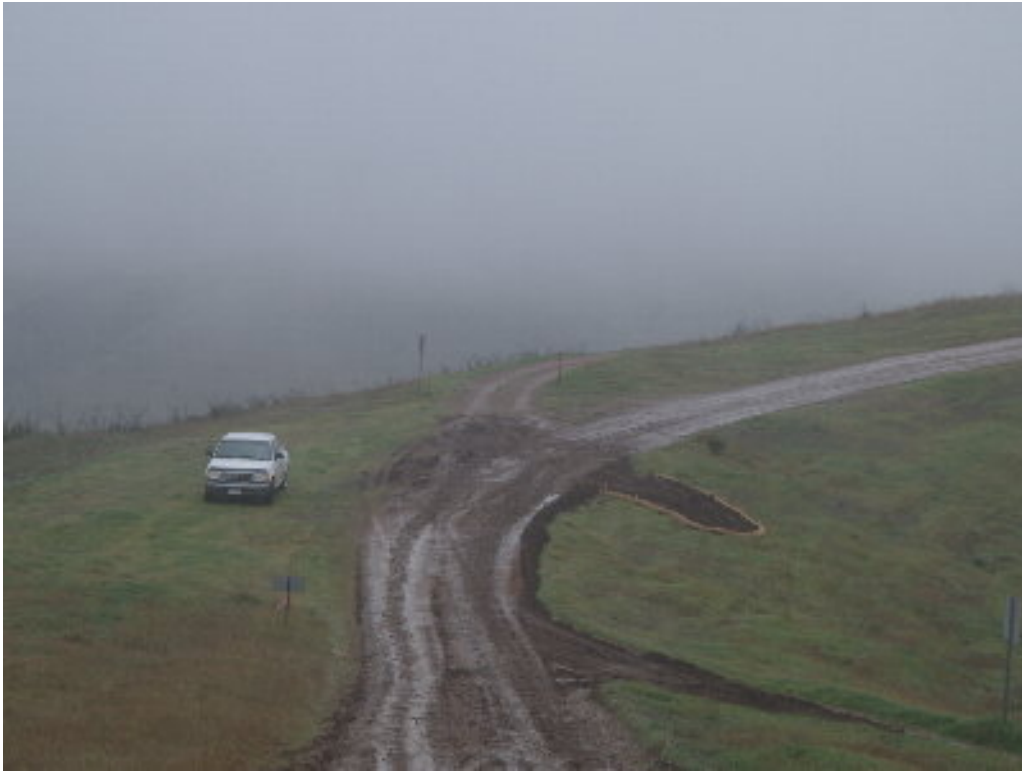
Figure 3 – The contractor worked on the access road to Fanita Junction and created erosion and sediment issues that were addressed by Essex and SDG&E.
