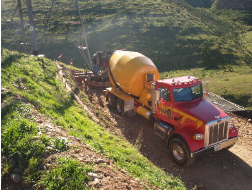
Figure 1 – The PAR concrete crew worked on pouring one of the foundations covered under NTP #3, on Miramar, during the subject week.
