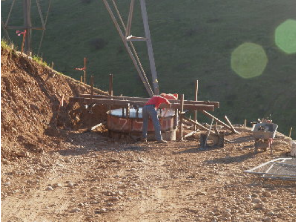
Figure 2 – The PAR concrete crew finished the surface of the foundation on Miramar.
