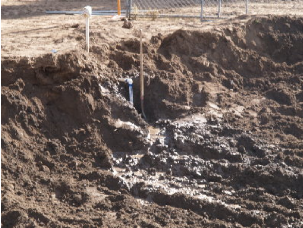
Figure 5 – The crew at Tower Site 1210 worked to restore water service to the residence adjacent to the excavation.
