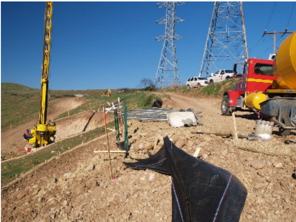
Figure 6 – Silt fencing backed by steel T-posts was used at Tower Site 621 to control rocks and other spoils during drilling.
