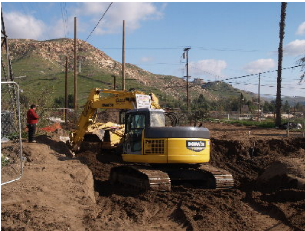
Figure 4 – The contractor continued work on compaction at Tower Site 1210 after the foundation was exposed for inspection. The current foundation will be removed below grade and the entire operation repeated.
