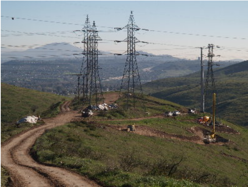
Figure 3 – The drilling activities continued at Tower Site 601. Crews worked to complete the work prior to the January 5 deadline for work on Miramar. Note that the spoil piles have been recovered and the roads watered.
