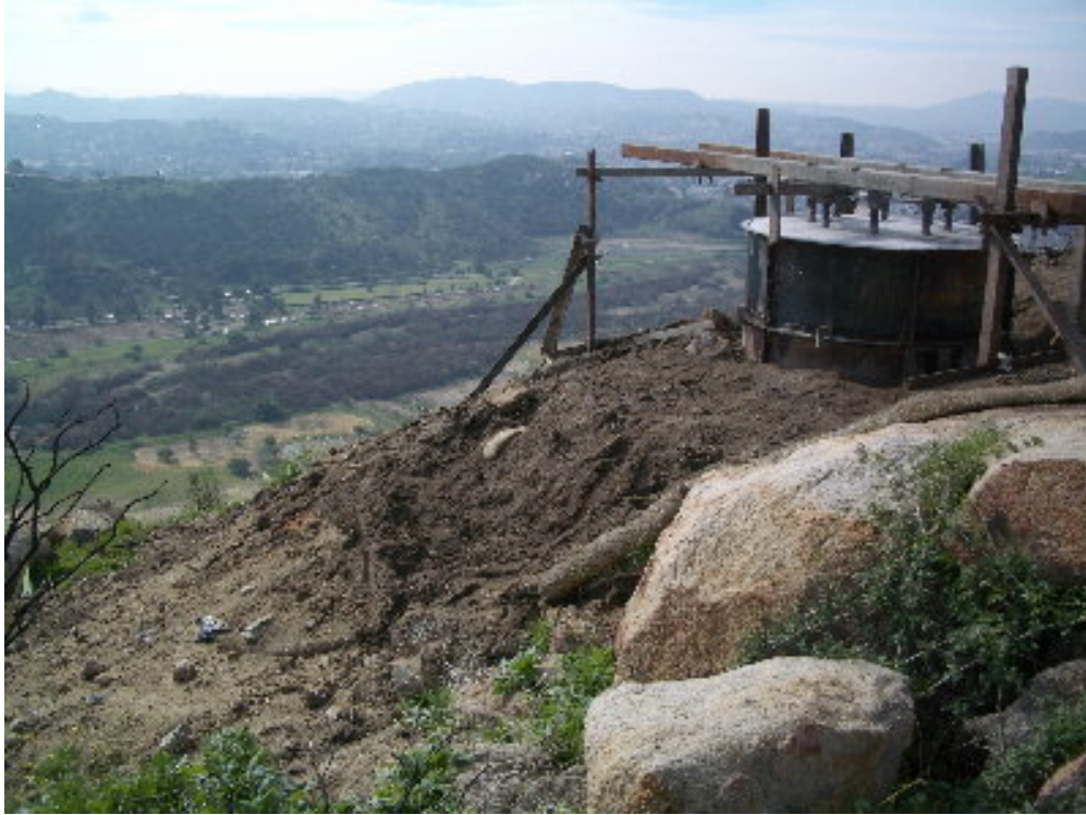
Figure 1 – Loose material at Tower Site 1180 needs to be stabilized prior to the predicted storm.
