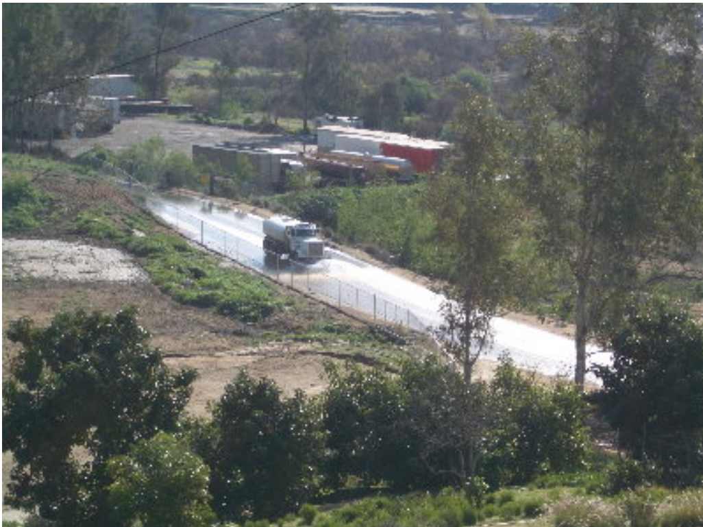
Figure 4 – The water truck was used to clean sediment transported onto the public road.
