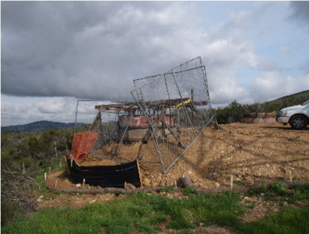
Figure 5 – Upon completion of the excavation, silt fencing was placed correctly at Pole Site 20.
