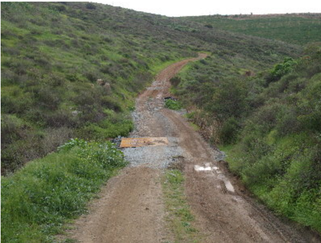
Figure 4 – One plate was placed on the access road to Pole Sites 10 and 20 to allow safe passage over the cut.
