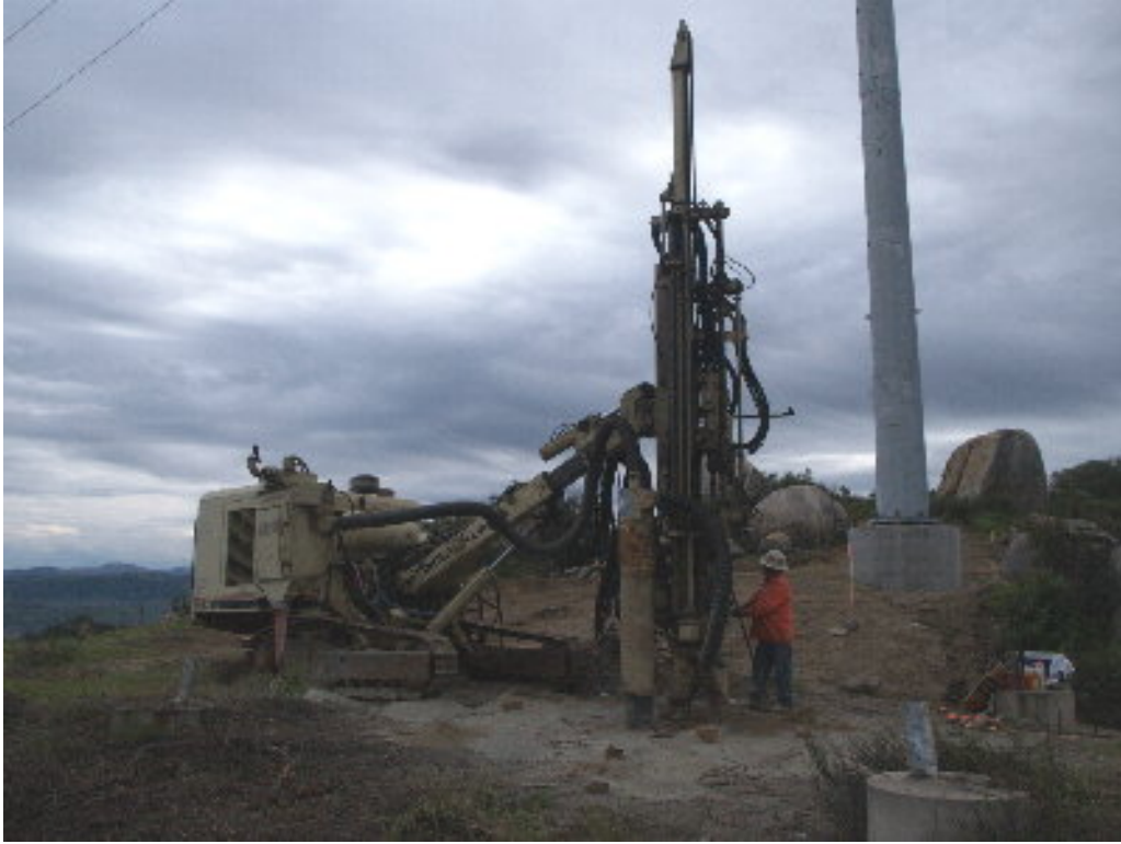
Figure 1 – An operator tested for rock prior to the drilling adjacent to Pole Site 1300.
