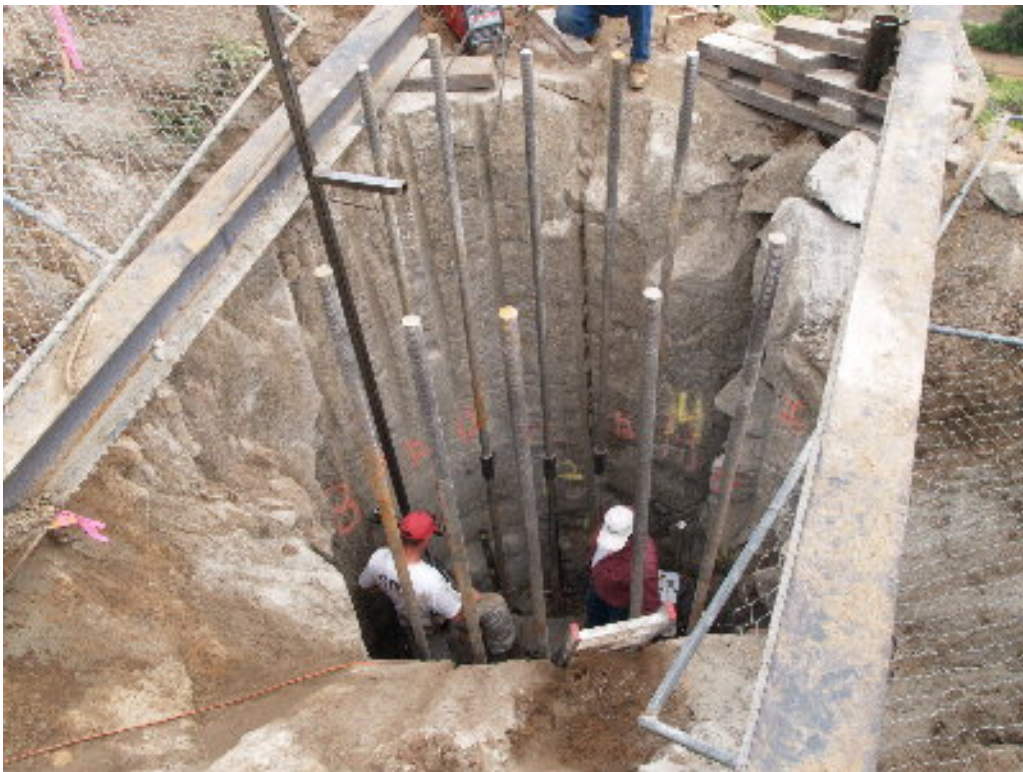
Figure 2 – A testing crew worked to check the strength of the micro-piles at Pole Site 1160.
