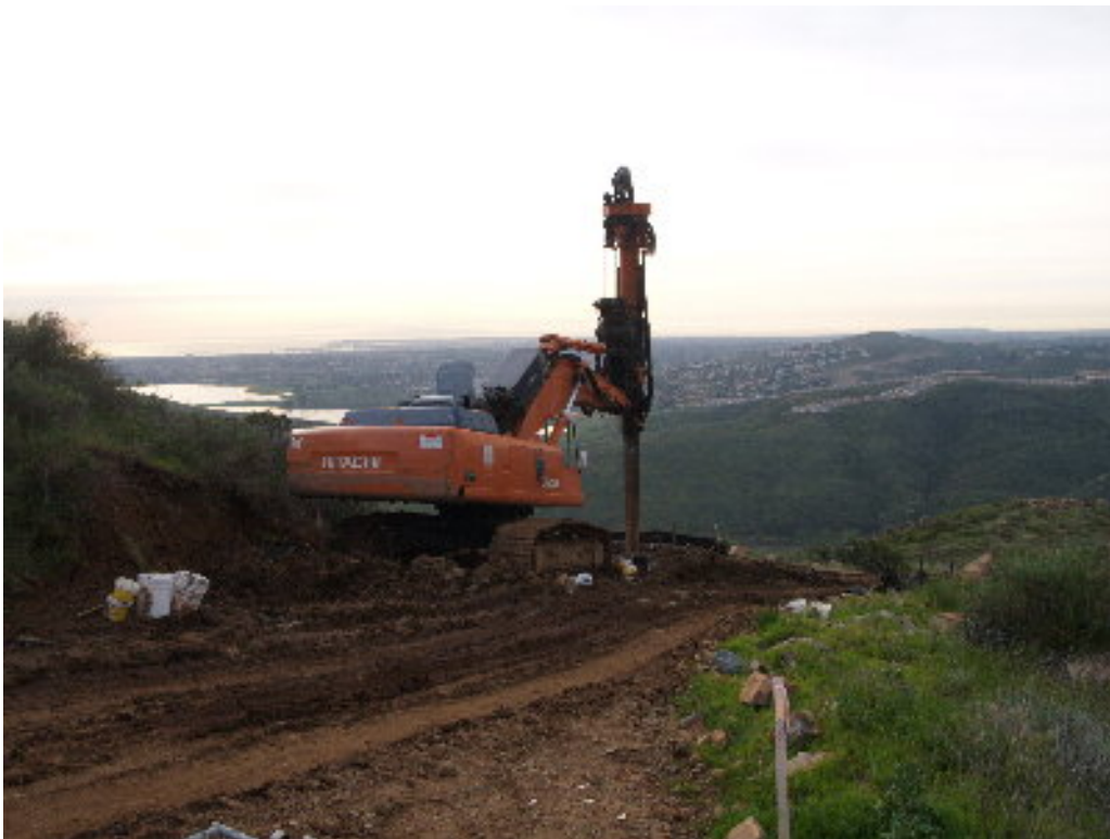
Figure 4 – A smaller drill was having problems with the hard material at Pole Site 171.
