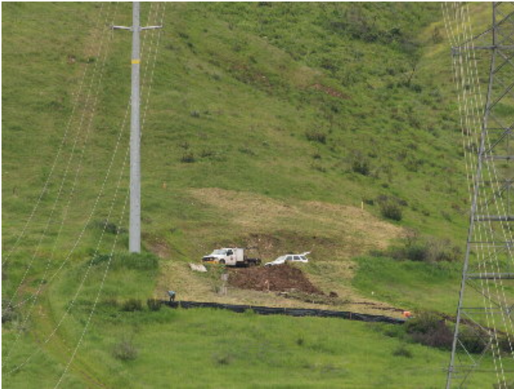
Figure 3 – A Wilson crew installed silt fencing adjacent to Pole Site 1330 after a new pad was graded for the 230 kV foundation.
