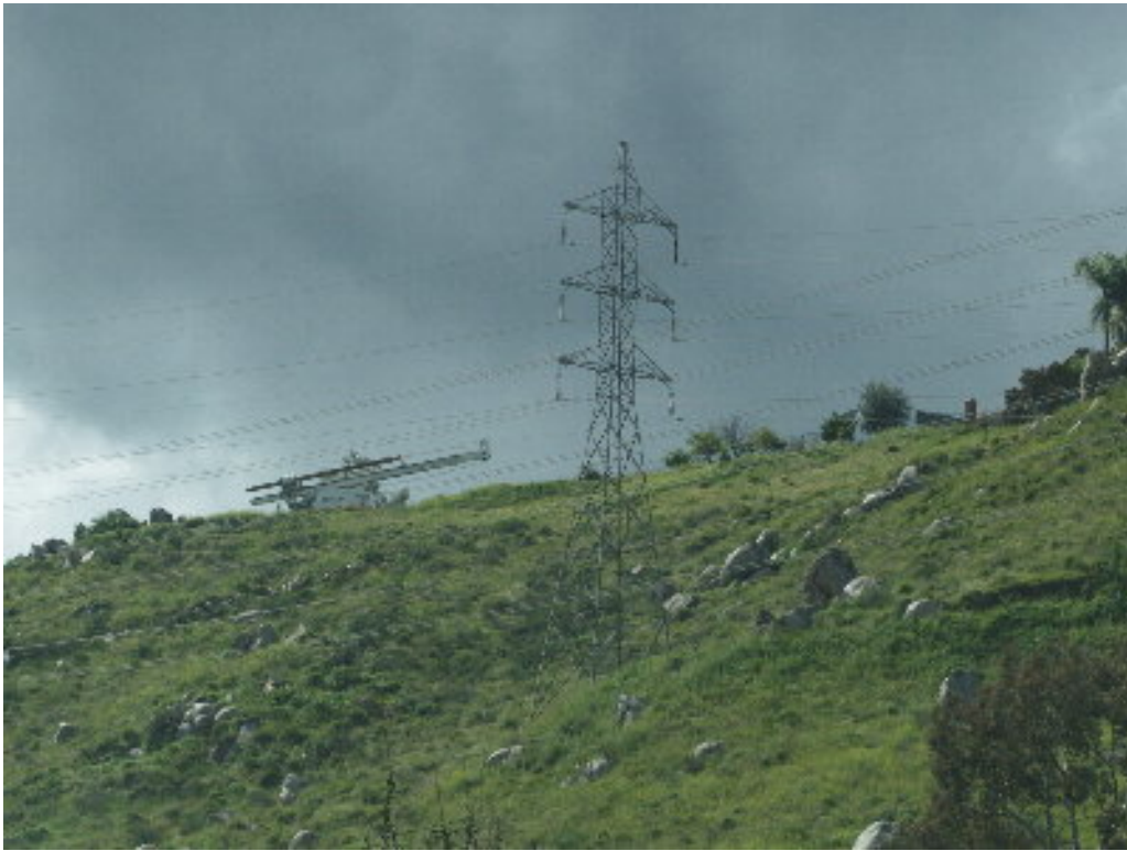
Figure 3 – The drilling at Pole Site 481 was completed and the Madco drill was removed from the site.
