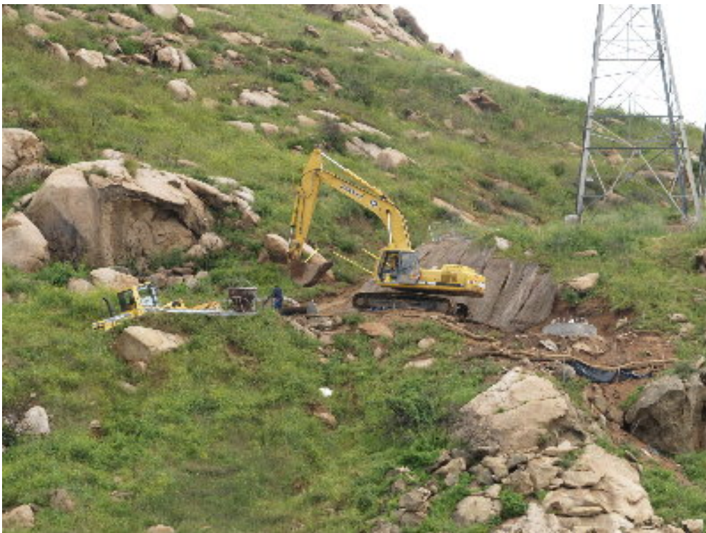
Figure 2 – The crew at Pole Site 1160 cleaned up after the pour and prepared for the sky crane with the lower pole section.
