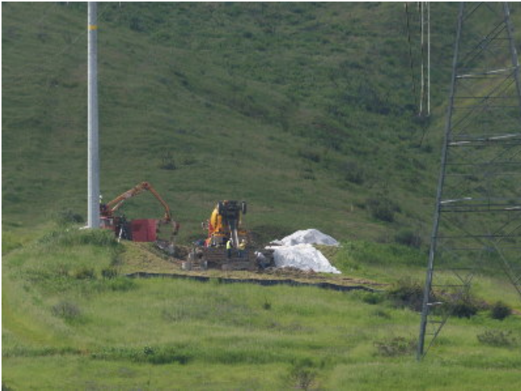
Figure 7 – The permanent 230 kV foundation for Pole 576650 was poured during the site visit.
