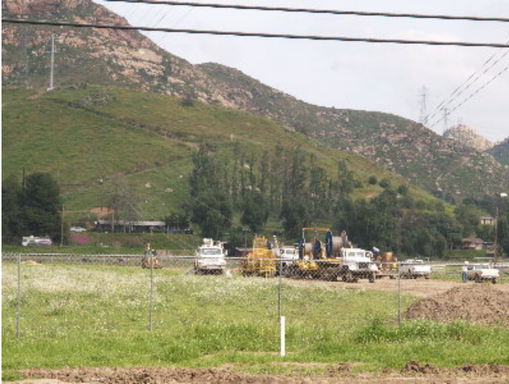
Figure 1 – The stringing operation set up across from Pole Site 1210 and pulled cable to Pole Site 1140.
