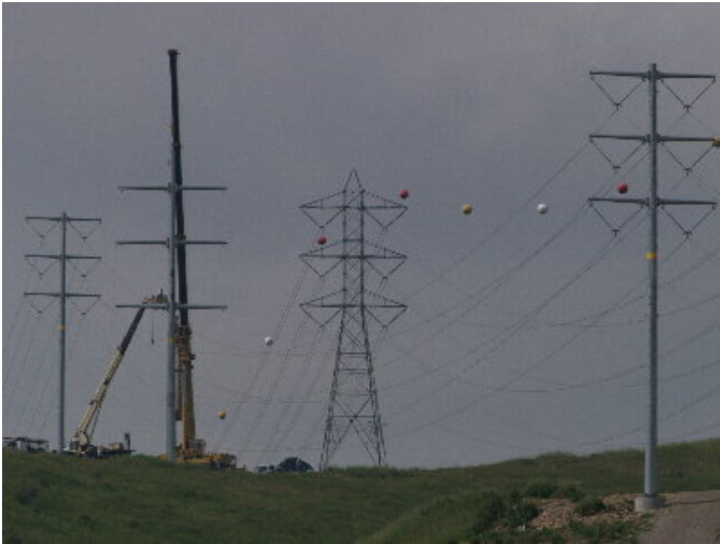
Figure 9 – Crews secured the upper section of the permanent 230 kV Pole 871862 once it was set in place.
