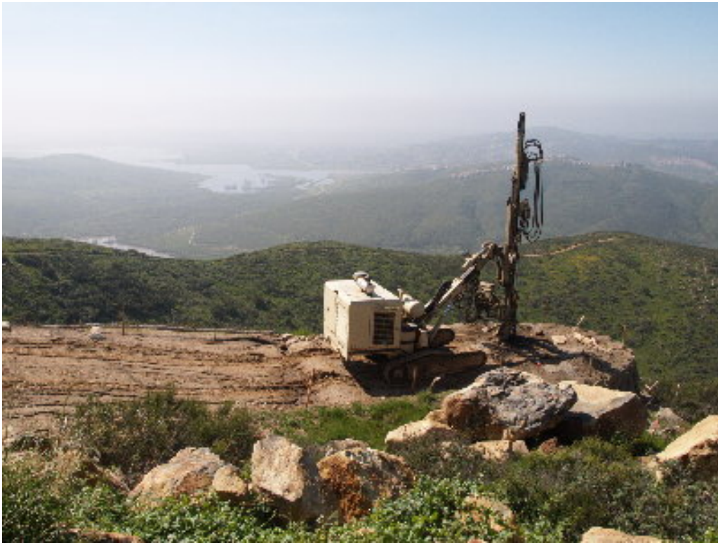
Figure 6 – A small drilling machine worked to prepare Pole Site 182 for the main drilling.
