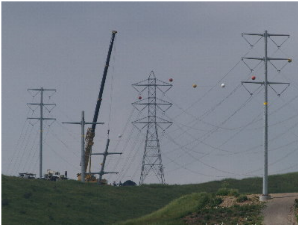
Figure 8 – The upper section of the permanent 230 kV Pole 871862 was set during the site visit.
