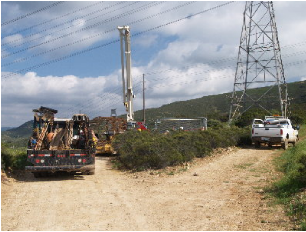
Figure 5 – The concrete crew moved into Pole Site 191 after initial problems getting the truck up the access road.
