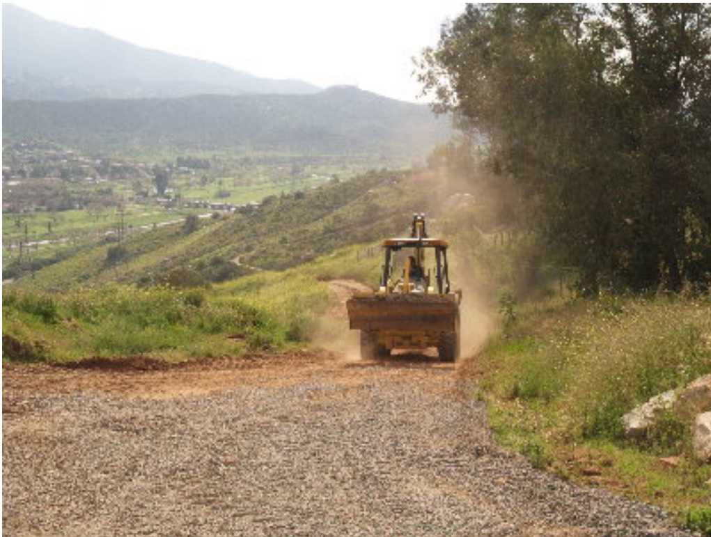
Figure 2 – The spoil removal operation at Pole Site 481 caused excessive fugitive dust that left the right-of-way.
