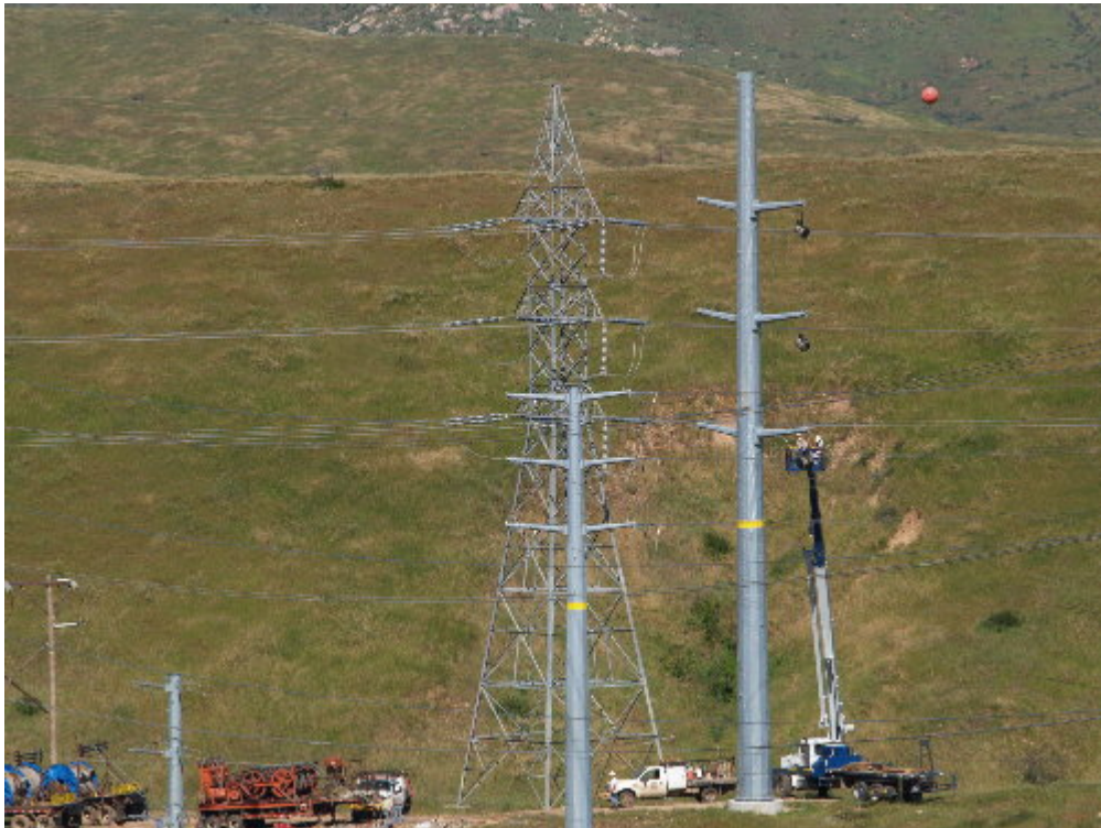
Figure 6 – Wilson crews worked at Fanita Junction to prepare for the pulling of conductor.
