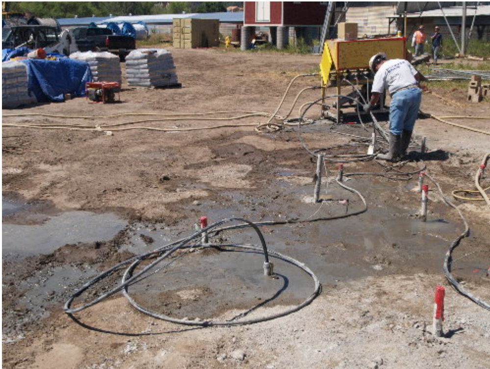
Figure 4 – Specialized equipment was used to pressure grout the annular spaces around the foundation at Pole Site 1210.
