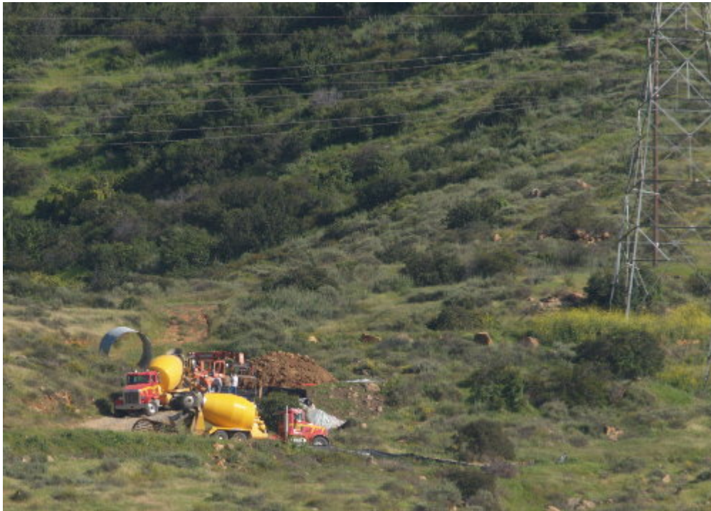
Figure 3 – Trucks delivered grout up the narrow access road to Pole Site 132 to stabilize the collapsed hole for drilling.
