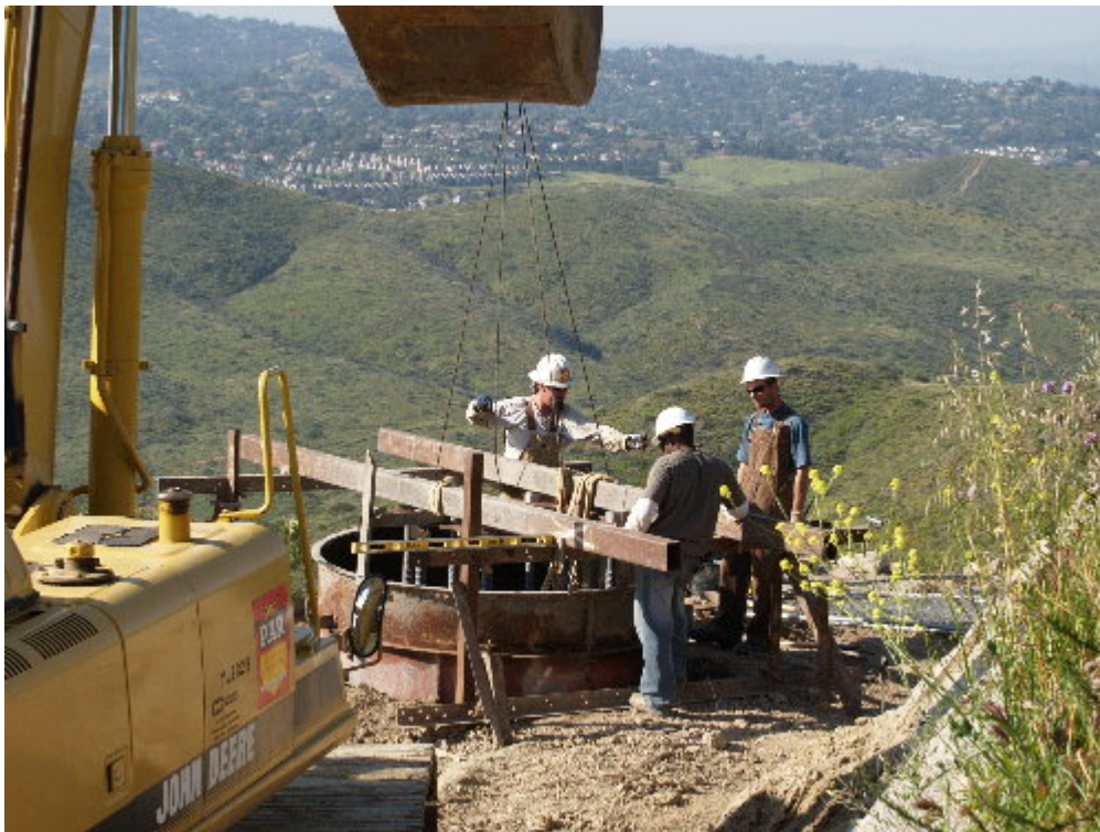
Figure 2 – PAR worked at Pole Site 181 to set the rebar cage and anchor bolts in preparation for pouring concrete.
