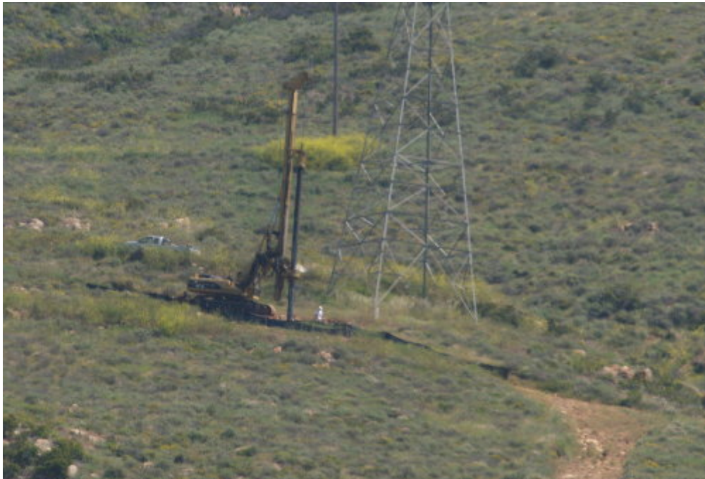
Figure 4 – The Woodward drilling crew worked at Pole Site 30 to complete the final 138 kV foundation excavation on the project.
