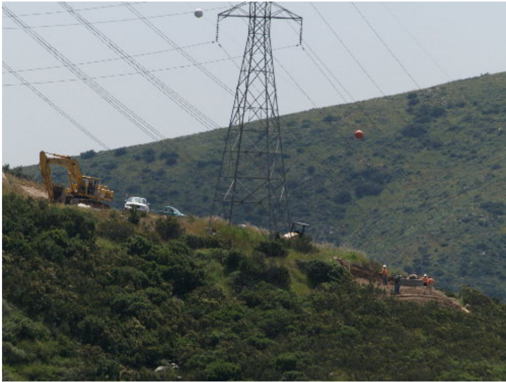
Figure 5 – The PAR grading crew worked with the Testing Engineers inspector at Pole Site 161 to repair the pad.
