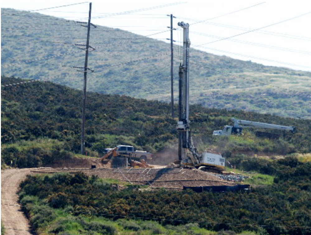
Figure 2 – The Magco drilling crew worked to finish the foundation at Pole Site 65-10.
