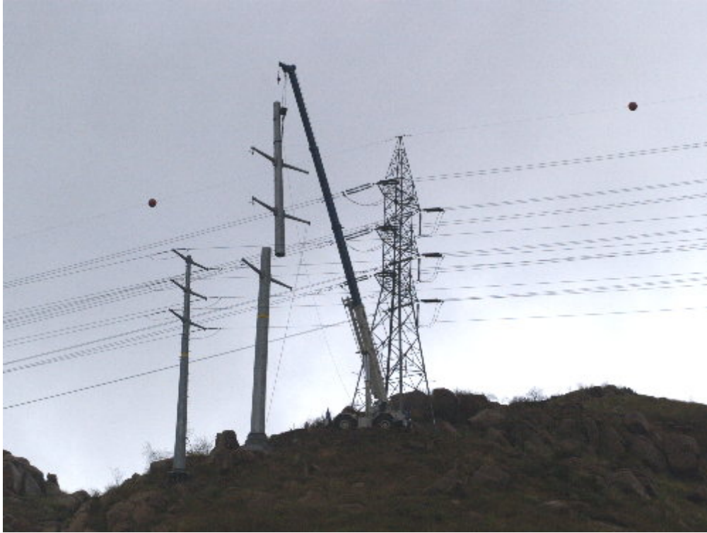
Figure 1 – The Wilson crew worked on setting the upper section of Steel Pole 576666.
