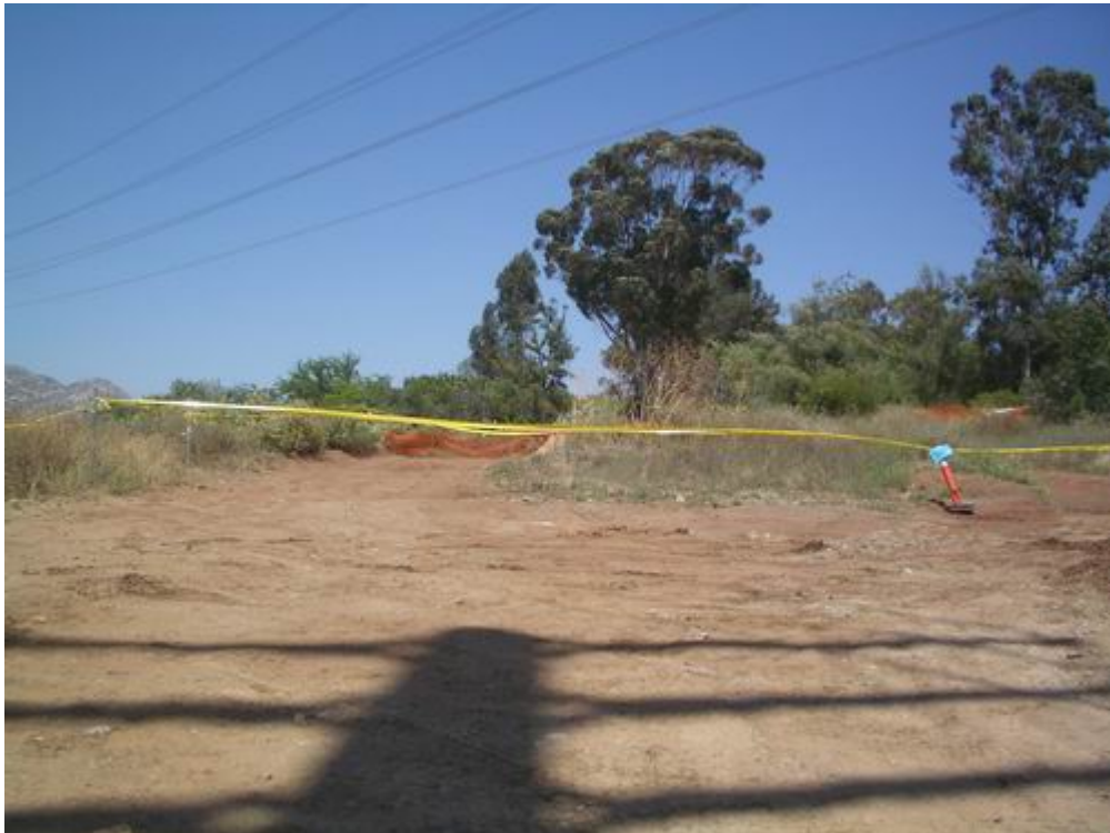
Figure 4 – The Essex EI has placed exclusion fencing and signs around the sensitive bird nesting sites above the Los Coches Substation.
