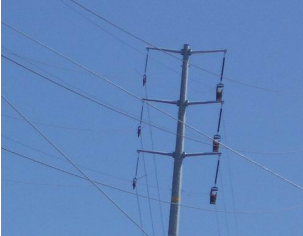
Figure 1 – The bundled conductor travelers can be seen on the right arm of the steel pole at Pole Site 20.
