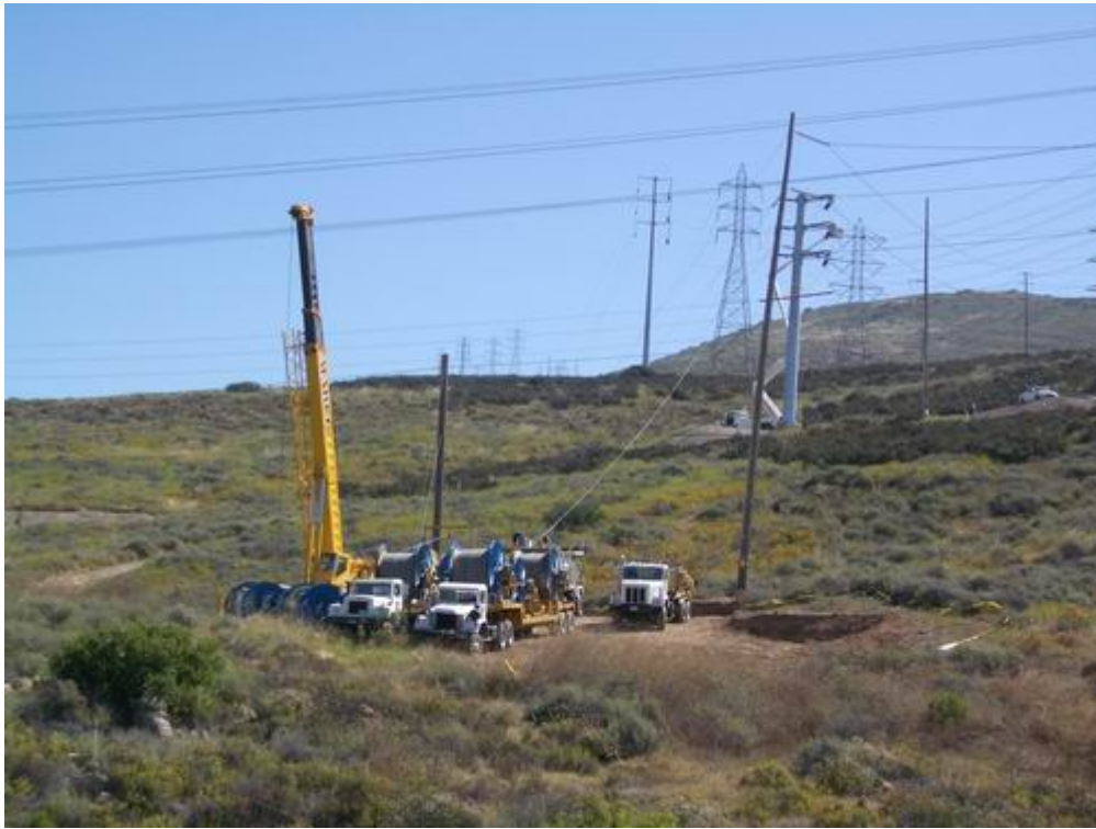
Figure 3 – The PAR stringing crew worked to pull conductor between the stringing sites at Pole Site 10 and Pole Site 100.
