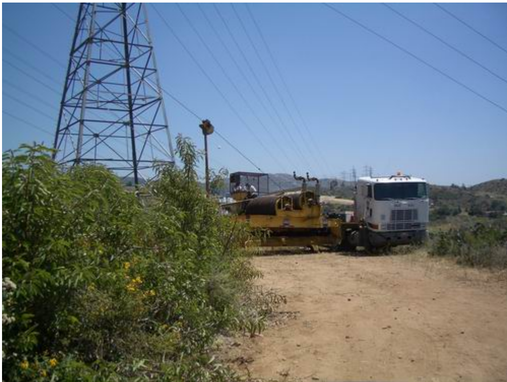
Figure 2 – The Wilson stringing crew pulled cable from above the Los Coches Substation.
