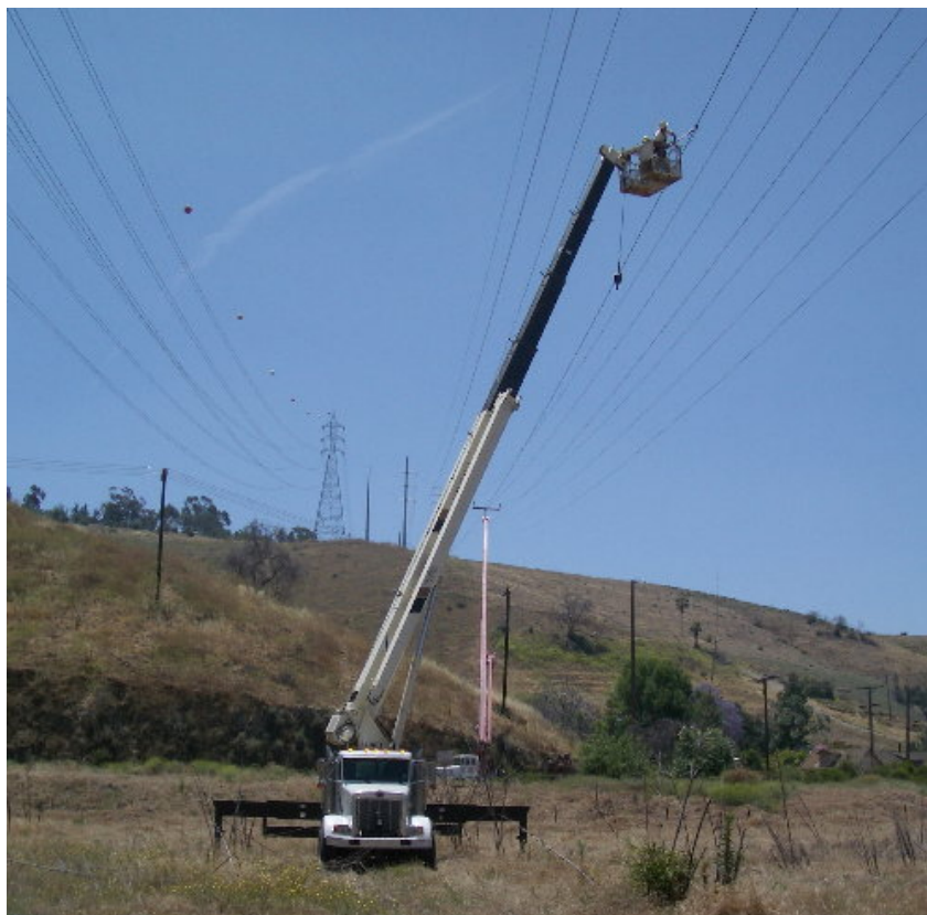
Figure 3 – Wilson and SDG&E inspecting the damaged conductor off El Monte Road.
