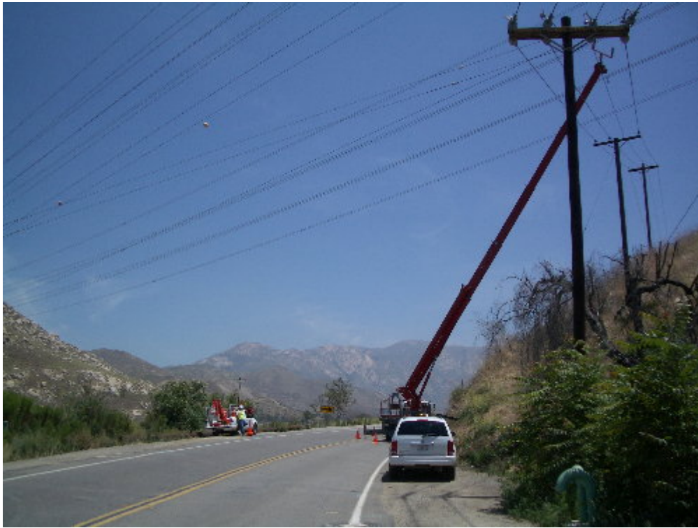
Figure 4 – Temporary protection of the distribution line on El Monte Road during inspection of the damaged conductor.
