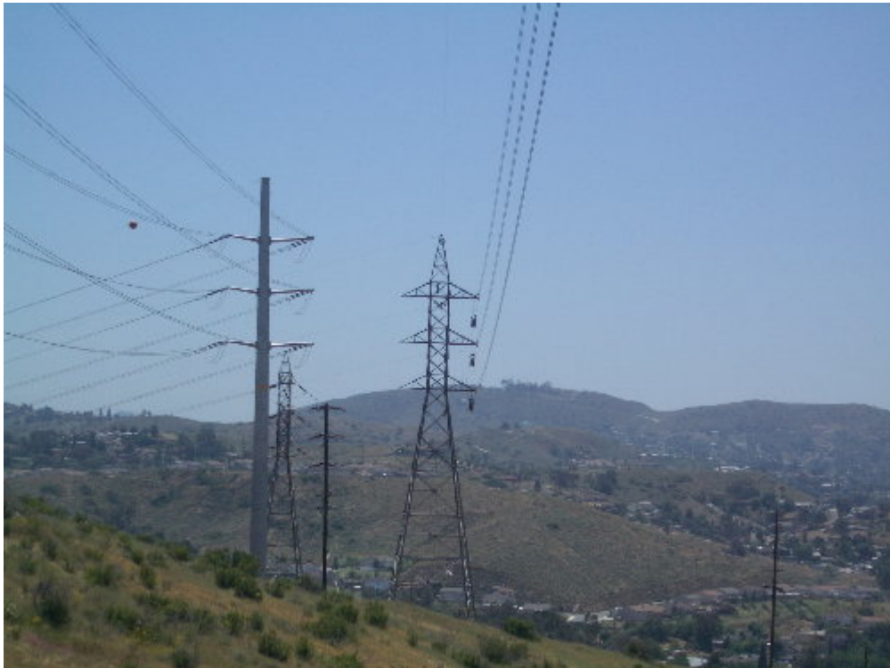
Figure 5 – End of the permanent 230 kV conductor above the Los Coches Substation.
