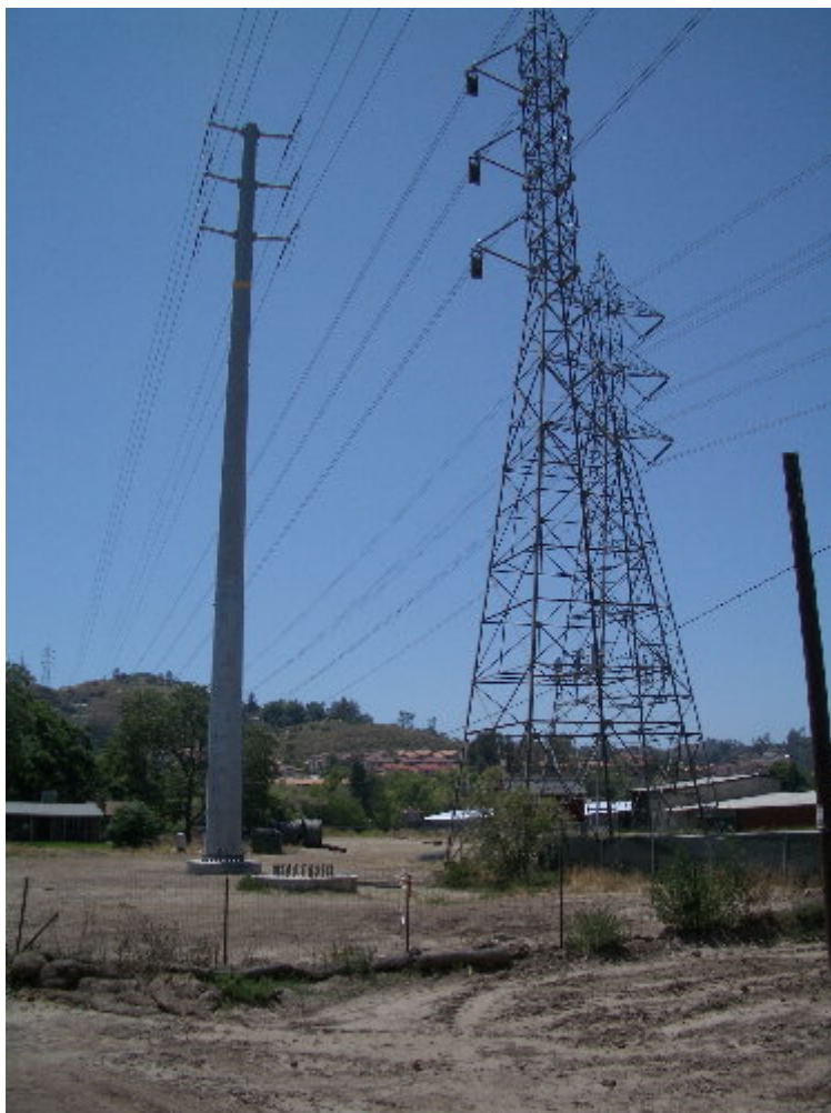
Figure 1 – The steel pole was relocated to the new foundation during a planned outage at Pole Site 1210. The bad foundation is in the foreground.
