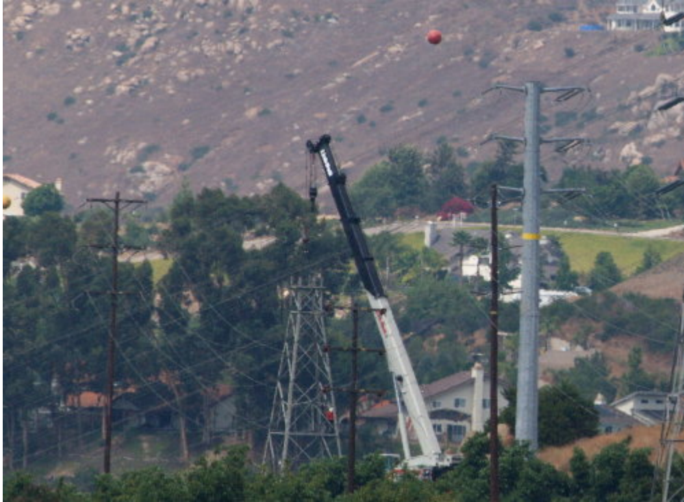
Figure 1 – The Wilson crew worked south of Interstate 8, dismantling the top of the existing lattice tower.
